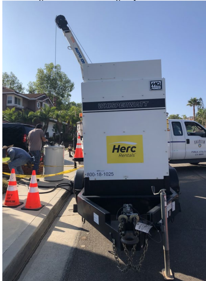
Figure 17: APU Emergency Generator
