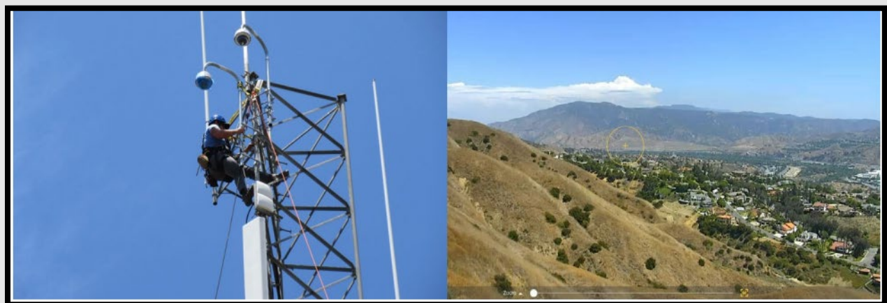
Figure 6: High Resolution Camera Installation and Camera Image Overlooking Anaheim
