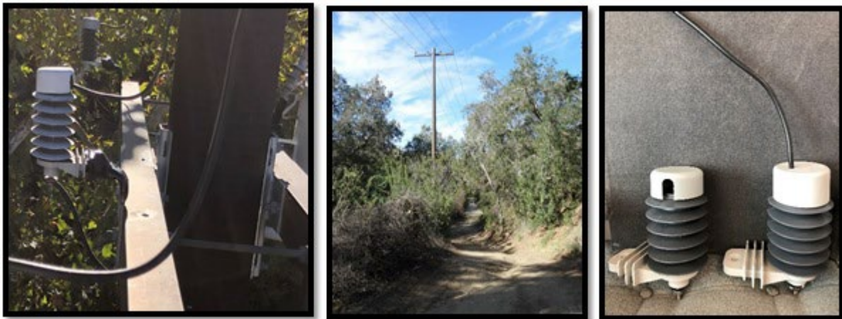
Figure 15: (a) Concealed Lightning Arrester (b) Ductile Iron Pole (c) Comparison of Lightning Arrester Models
