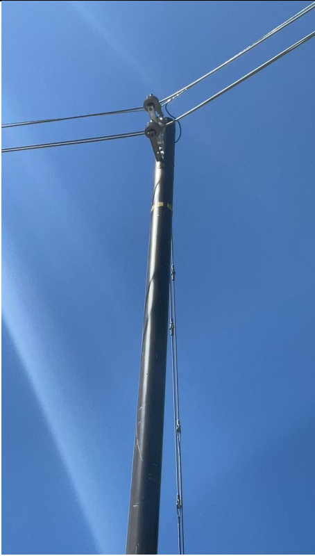
Item9IA3Img1: No Fuse Installed
