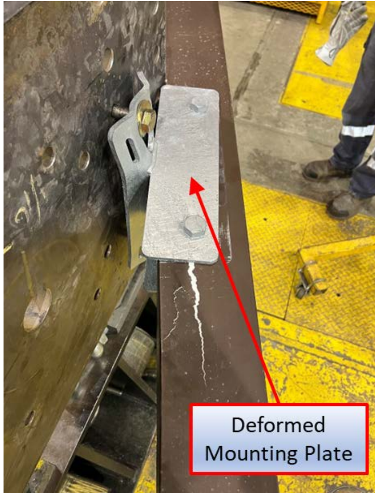
Figure E5. A representative post-test image showing typical deformation of the cross-arm mounting plate.
