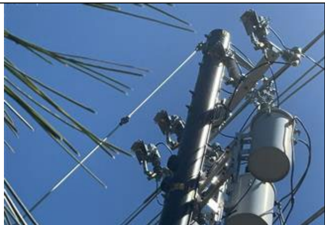
Item8IA3Img2: Missing fuse
