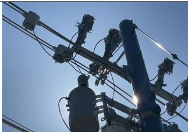
Item8IA3Img1: Missing one out of four expulsion fuses
