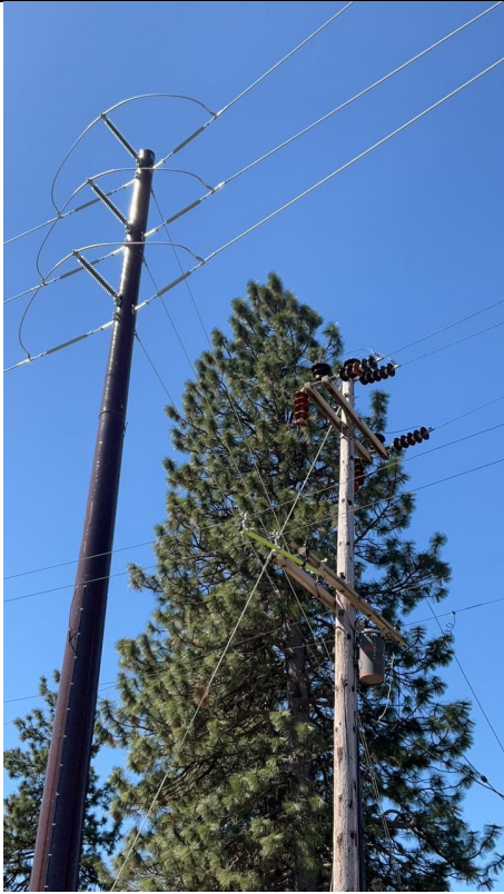
Item3IA1mg1: No fuse installed
