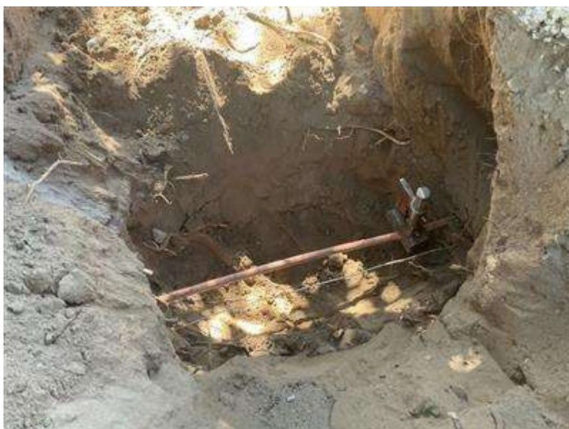
Photo 2 provided by Southern California Gas Company depicts the half-inch natural gas line. (Exh. 1.)
