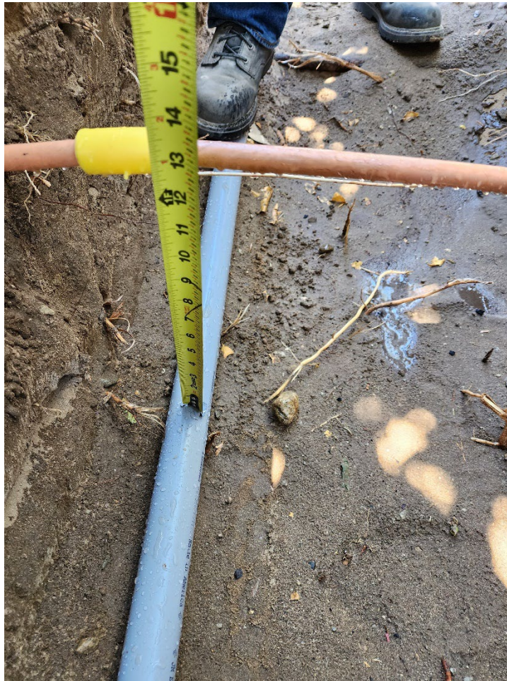
Photo 3 provided by ARM Construction depicts the half-inch natural gas line. (Exh. 4.)
