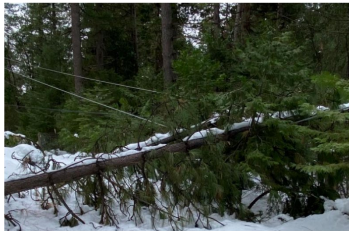
Figure 4: PG&E Covered Conductor Effectiveness – Example 3
