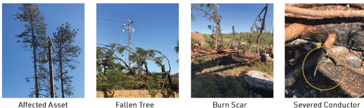
Figure 2: PG&E Covered Conductor Effectiveness – Example 1
