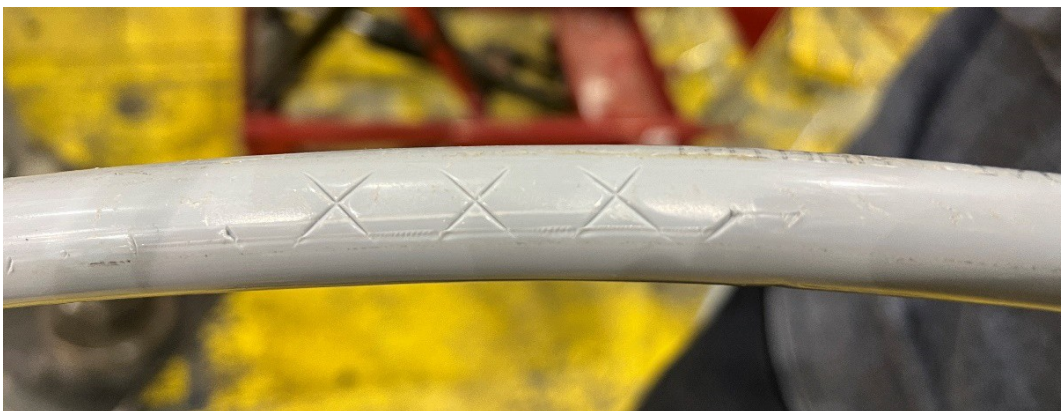
Figure 6-24: Sample 3.4.3 - 15 kV, 1/0 AWG ACSR Condition after Test
