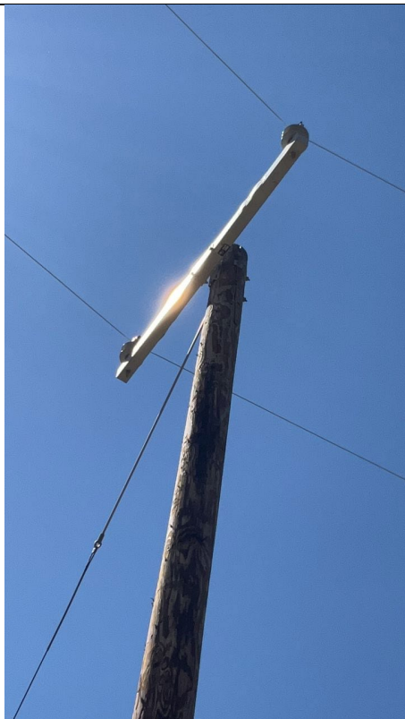
Item7IA1Img1: View of subject pole with no fuses.
