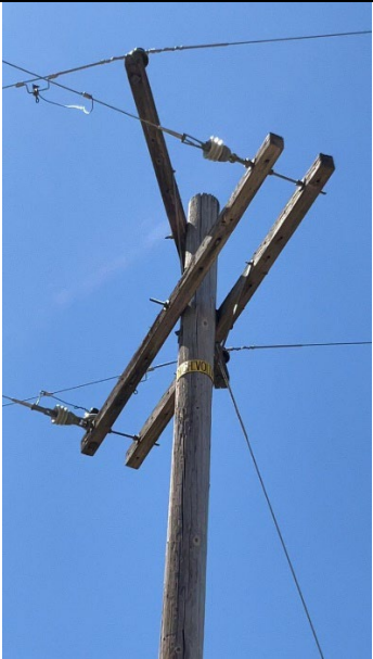
Item2IA1mg1: View of subject pole with no fuses.
