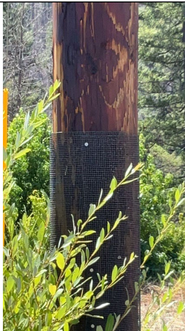
Item7GImg2: Pole ID is absent.
