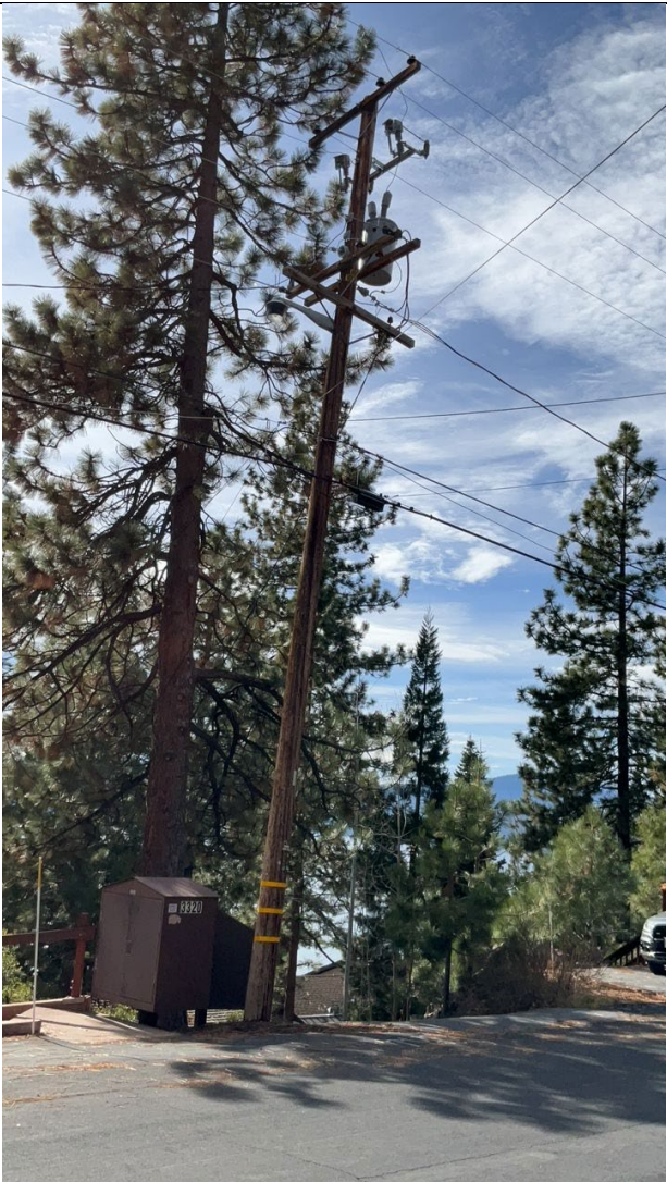
Item3GImg2: Overall pole.
