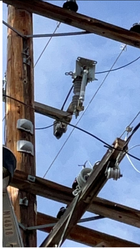
Item3IA1mg2: Close-up view of installed non-expulsion fuse indicating half the reported initiative work was completed.
