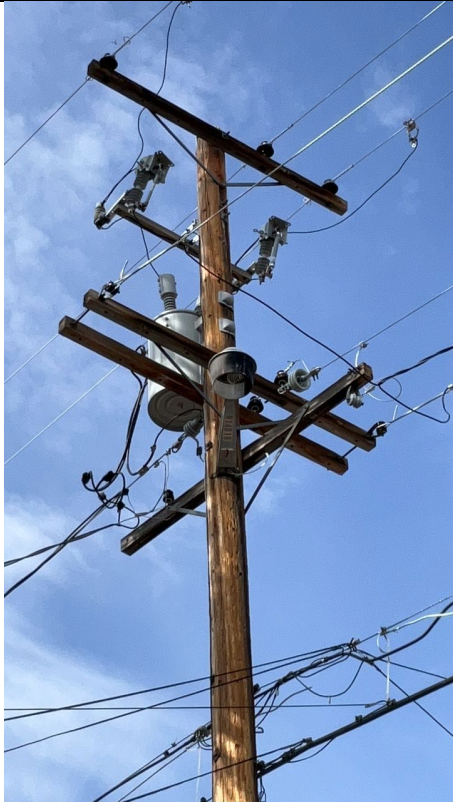
Item3IA1mg1: View of one expulsion fuse (left) and one non-expulsion fuse (right).
