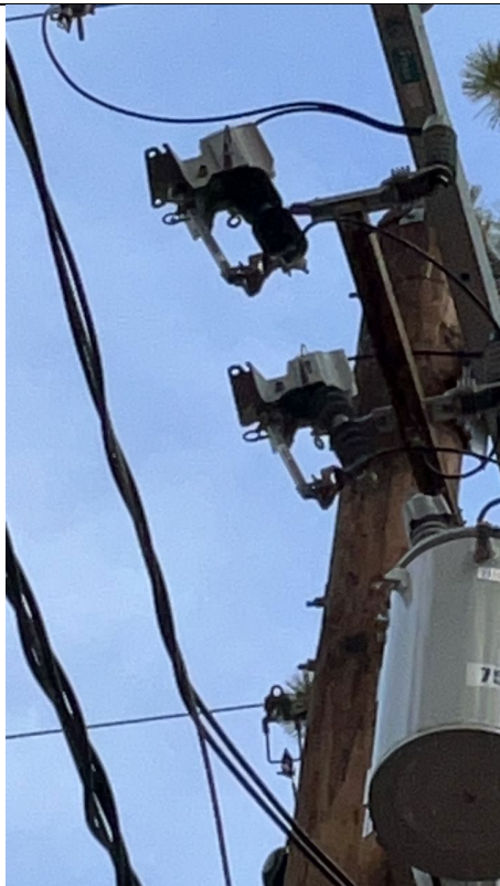
Item4IA1Img1: Close-up view of expulsion fuses.
