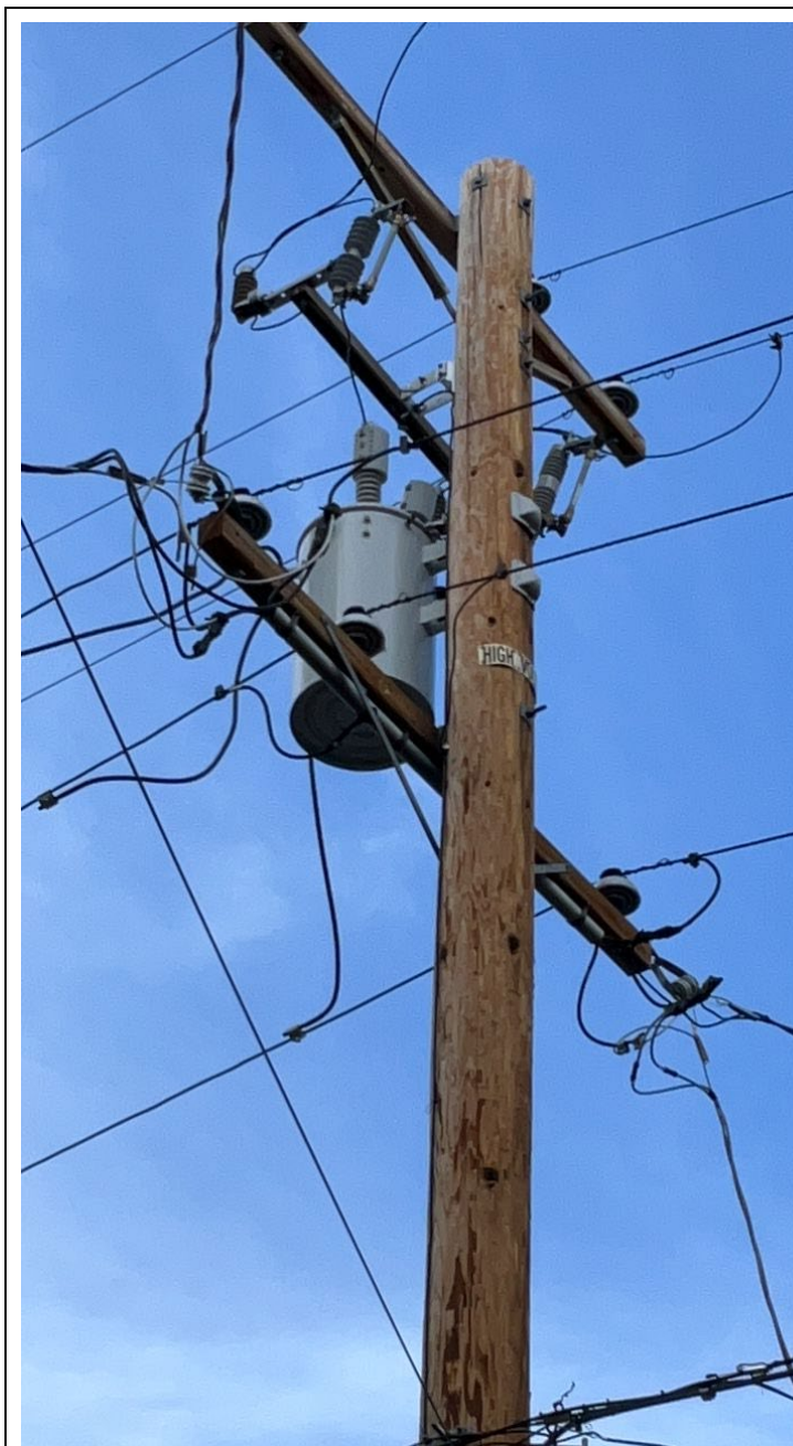
Item10IAimg1: View of two expulsion fuses.
