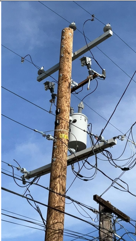
Item9GImg3: View of two expulsion fuses (open).
