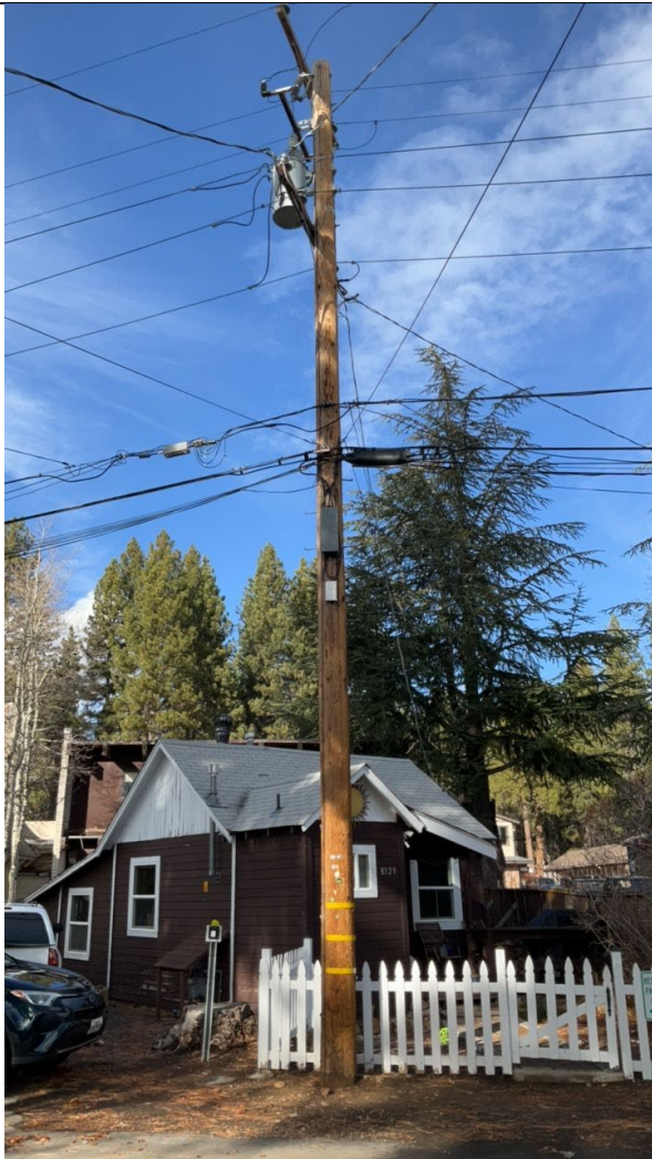
Item10GImg1: Overall pole.
