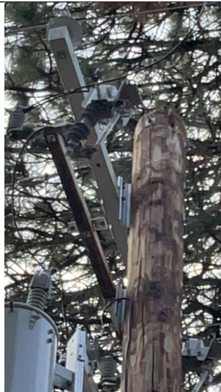
Item4IA1Img2: Close-up view of expulsion fuses.
