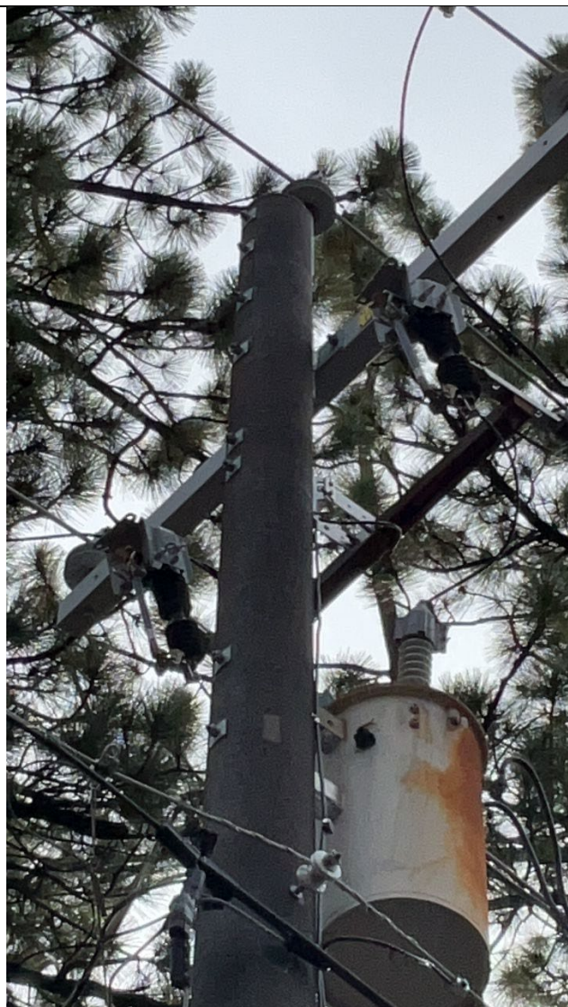
Item1IA1Img2: Close-up view of expulsion fuses.
