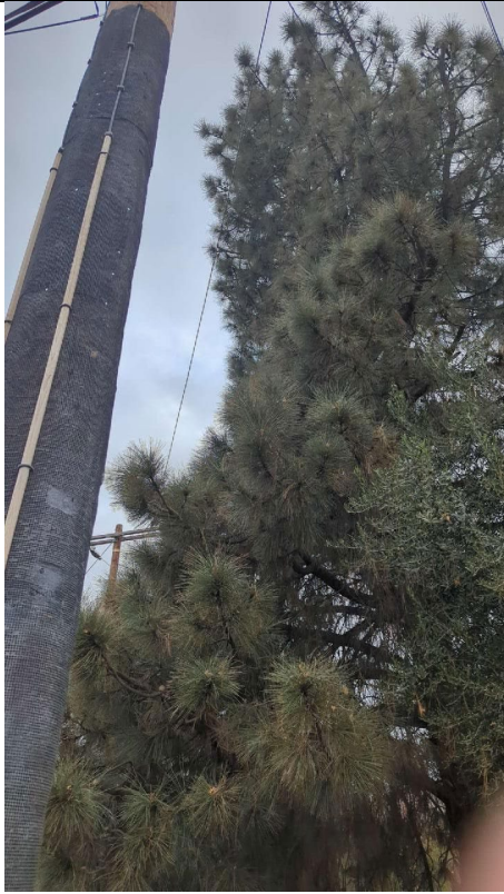
Item4IA2Img1: View of vegetation within four feet from the distribution line.
