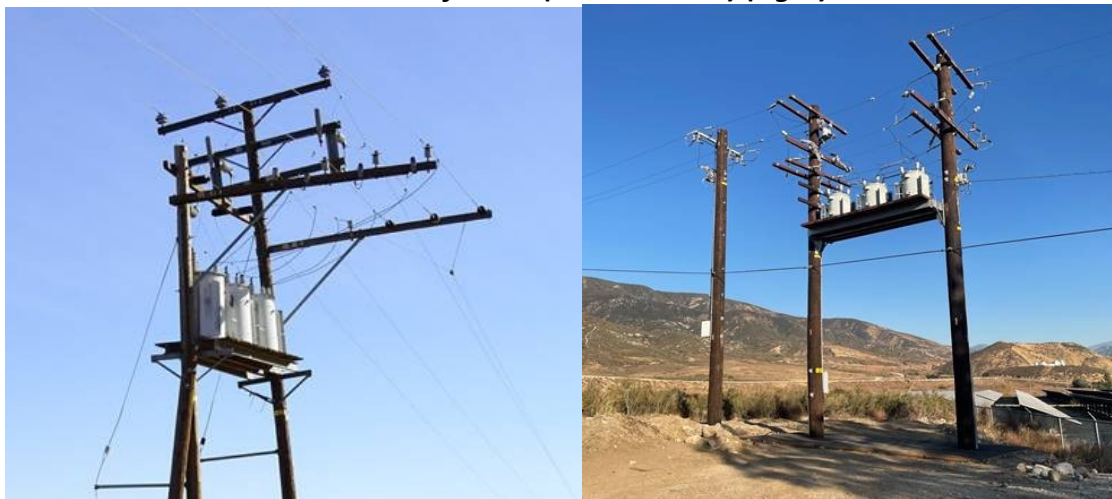
Figure SCE 8-12 - Pole Top Step Down (33kV to 12kV) Transformer (left) and Isolation (Iso) Bank Transformer (12kV to 12kV) (right)
