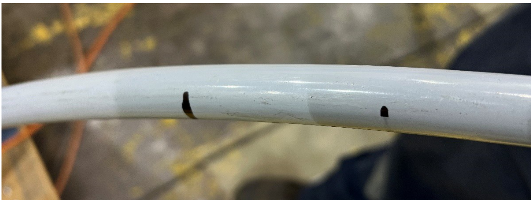
Figure 6-34: Sample 3K.1.3 - 17 kV, 1/0 AWG ACSR Condition after Test
