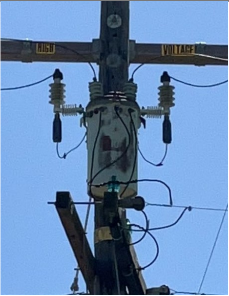
Item6IA21mg1: View of primary transformer bushings without wildlife covers.
