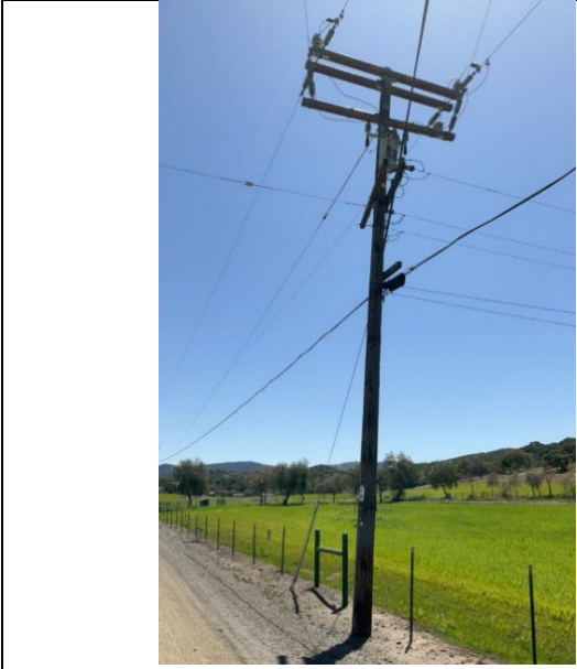
Item6G1mg1: Overall pole.
