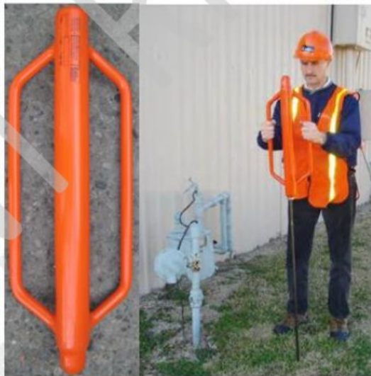
Image of slide hammer driving a probe rod from Southern California Gas Company procedures, Lobos Avenue (Atascadero) Gas
