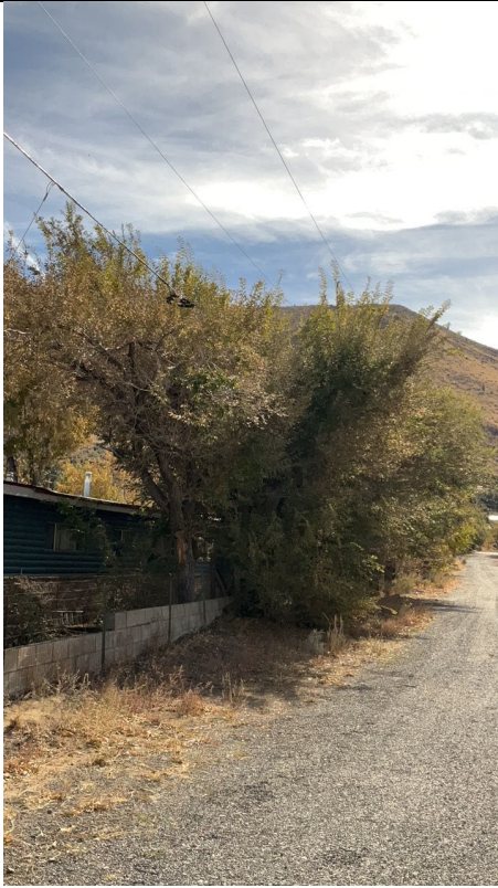
Item1Gimg3: West view of elm trees underneath the primary conductor.
