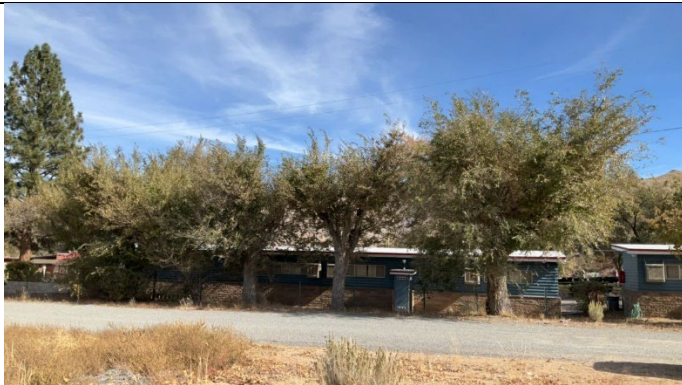
Item1Gimg5: Overview of clearances of the two elm trees growing underneath high voltage primary conductors. The two elm trees were measured at approximately three feet and five feet under primary conductors.
