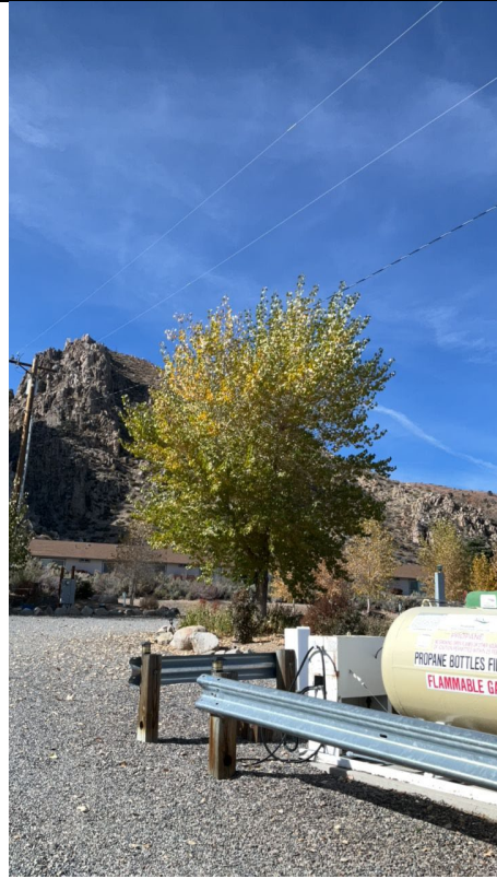
Item4IA1Img2: Secondary view of cottonwood tree within six ft of a primary conductor.
