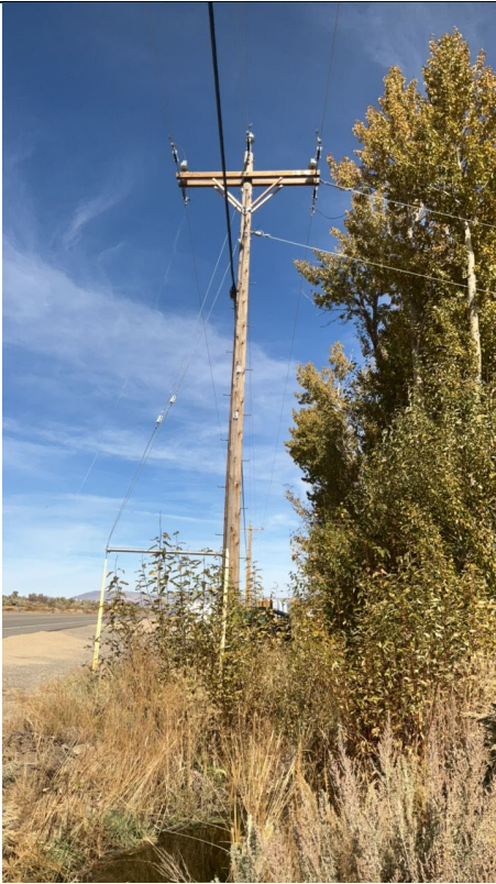
Item2G1mg2: Overall pole.
