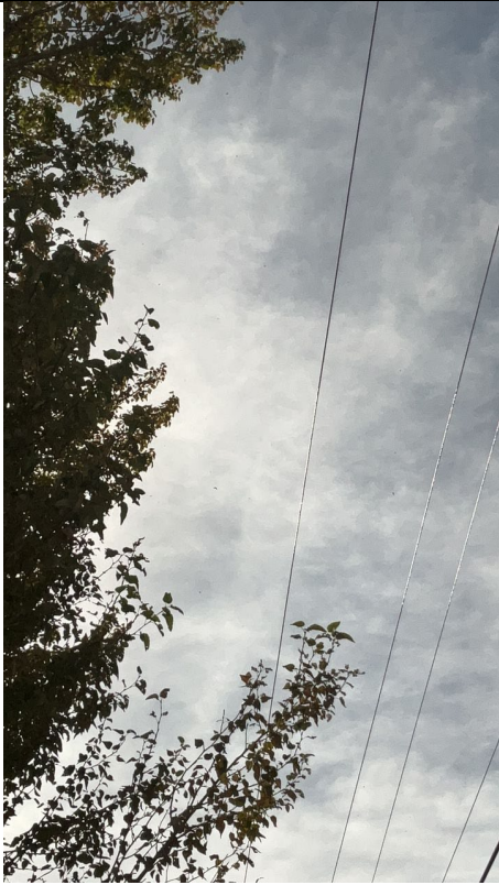
Item2IA1Img1: View of cottonwood limbs approximately four to five ft from a primary conductor.
