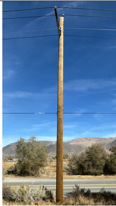
Item5GImg2: Overall pole.
