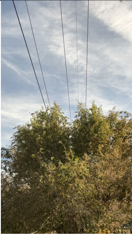
Item5IA1Img1: Front view of elm tree within five ft from a primary conductor.
