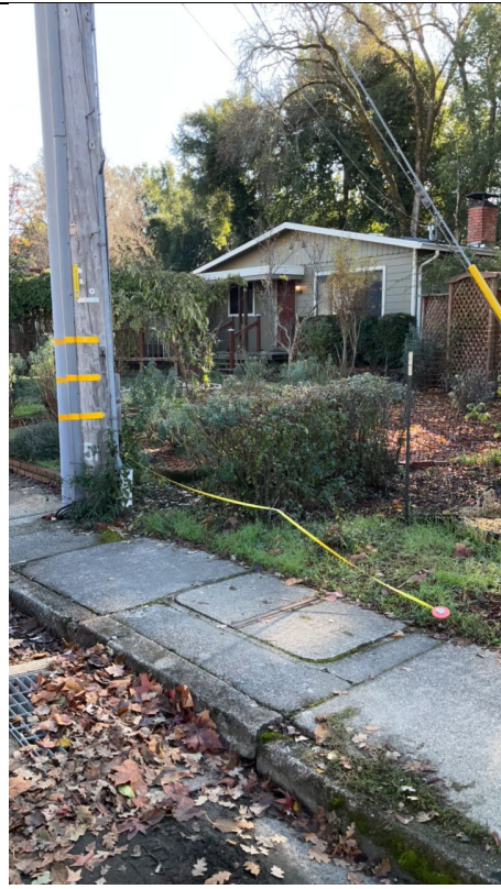
Item6IA1Img2: View showing live vegetation within 10-foot radial clearance. Tape measure at base of pole extends ten feet.
