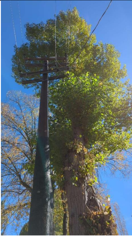
Item4IA1Img1: View of tree growing within three feet of bare conductors.
