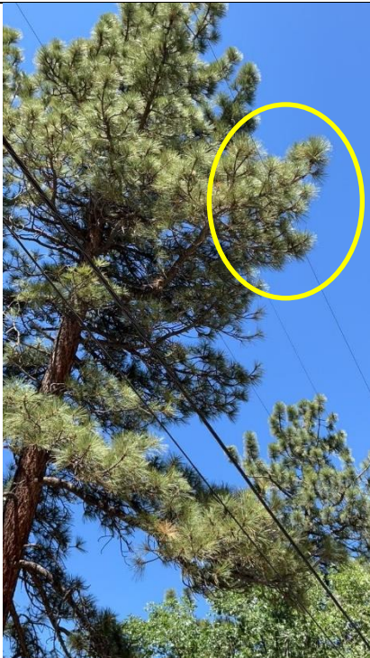
Item4VG4Img3: Third mid-span view of vegetation within minimum distance requirements of 4 feet to primary conductors
