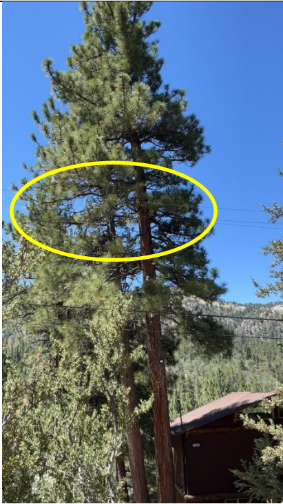
Item4VG4Img1: Mid-span, vegetation within minimum distance requirements of 4 feet to primary conductors
