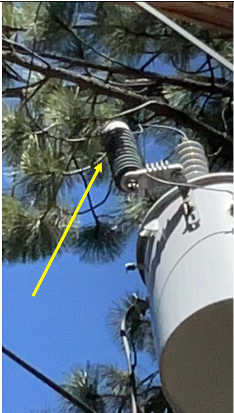
Item14CD3Img3: Burnt surge arrester, indicating possible arcing on the surge arrester
