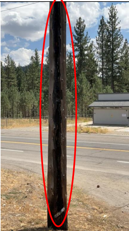
Item3PL2Img1: Fire damaged
