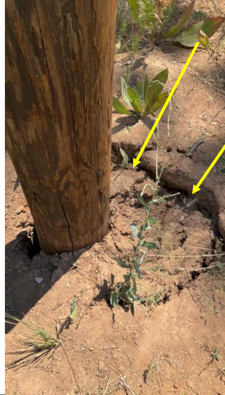
Item5IA2Img1: Possible material movement at the base of the pole
