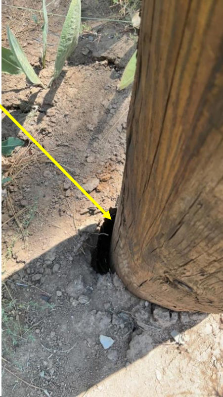
Item5IA2Img2: Hole at the base of pole that was not filled in or firmly set
