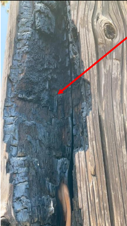
Item3PL2Img2: Fire hollowed out pole
