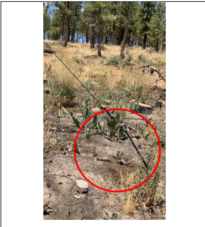
Item1GW1Img1: Guy anchor rod and strand vice pulled out of the ground
