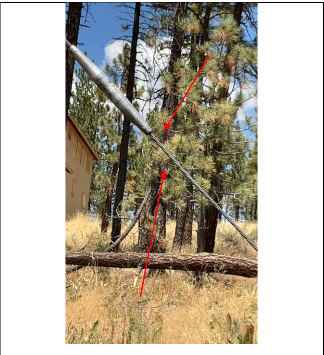
Item1GW1Img2: Evidence of Guy Wire having been exposed to fire
