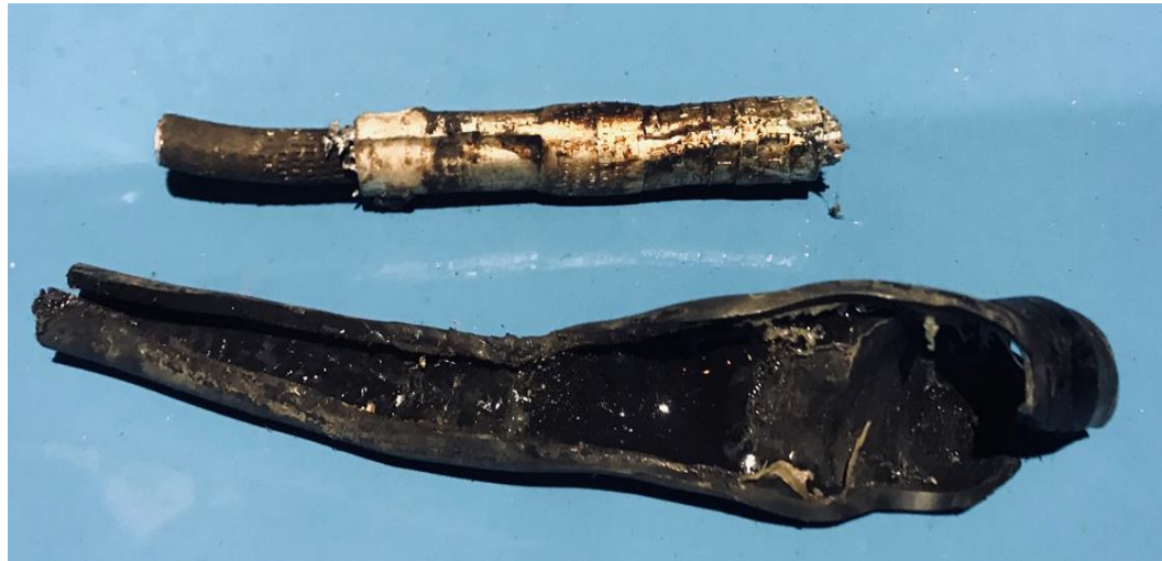
Photograph 1: Taken on June 22, 2020 of the secondary neutral splice with pin terminal connector (Top) and rubberized cover (Bottom) that was recovered by the troubleman
