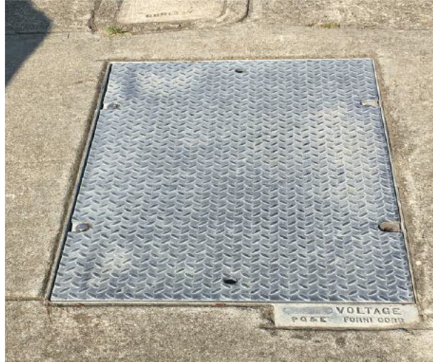
Photograph 4: Taken on October 4, 2021 of the secondary splice box lid
