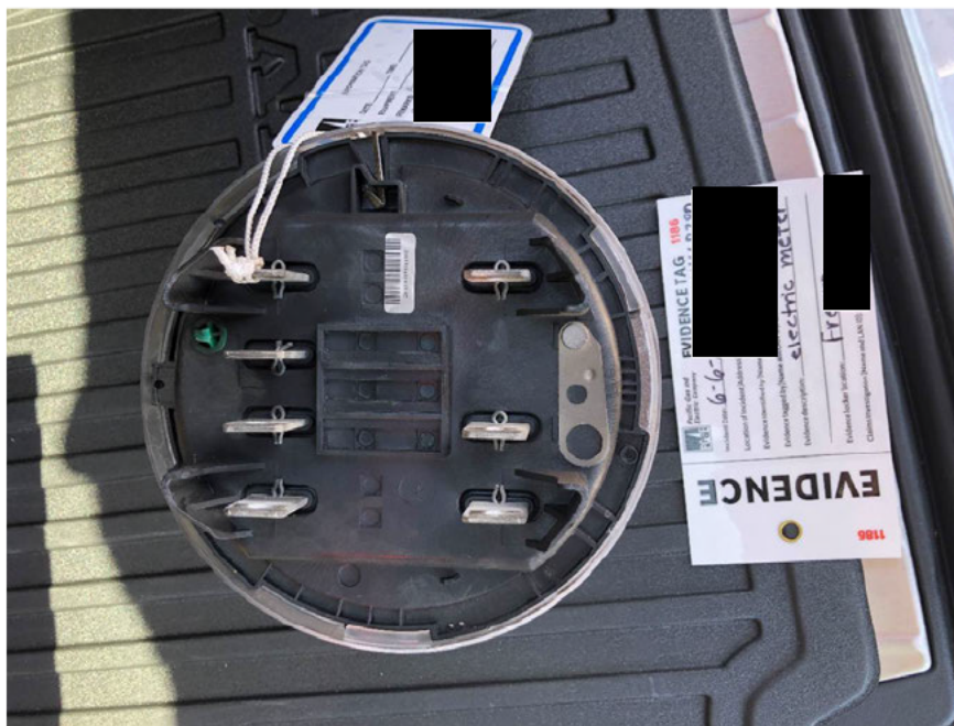
Figure 7: No damage to prongs of SmartMeter. Photo taken by Law Claims on June 25, 2021.
