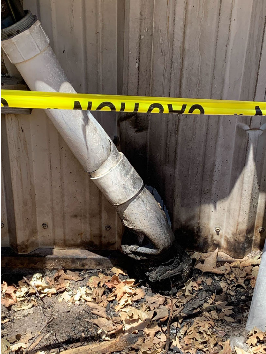
Figure 5: Crack on conduit exterior above joint. Photo taken by meter tech on July 1, 2021.
