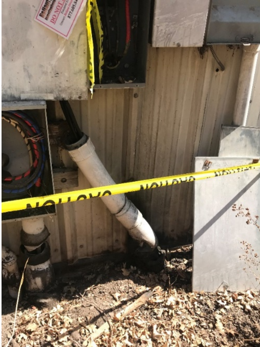
Figure 4: Service conduit–base melted from heat of fire. Photo taken during site visit on July 19, 2021.
