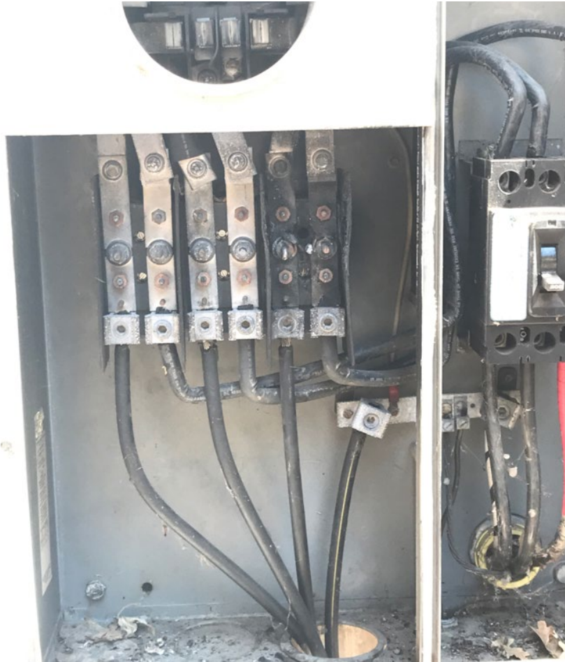
Figure 8: Terminal Block under meter – right side shows damage. Opening in bottom of panel is visible. Taken on site visit July 19, 2021.
