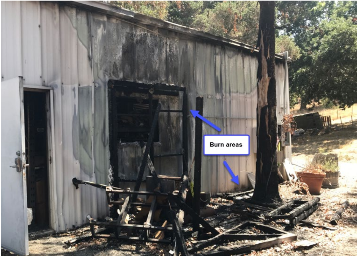
Figure 2: Exterior of Incident Location - charred area adjacent to AC unit and down along perimeter base of building. Customer panel on right side of building. Photo taken during site visit on July 19, 2021.
