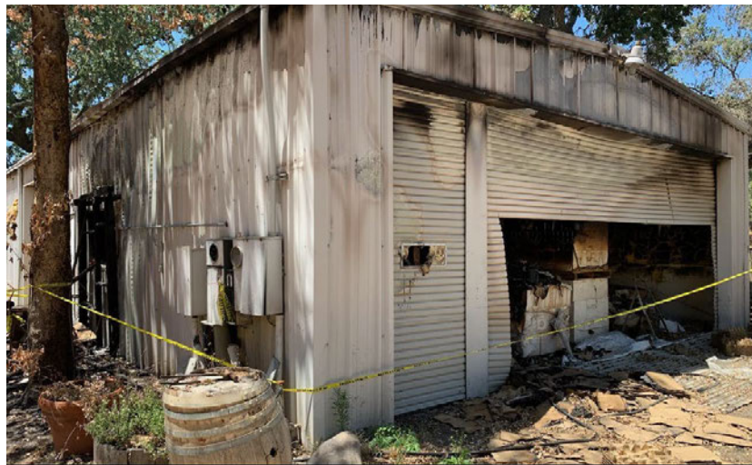
Figure 9: Roll up door accessed by first responders. Photo taken by meter tech on July 1, 2021.
