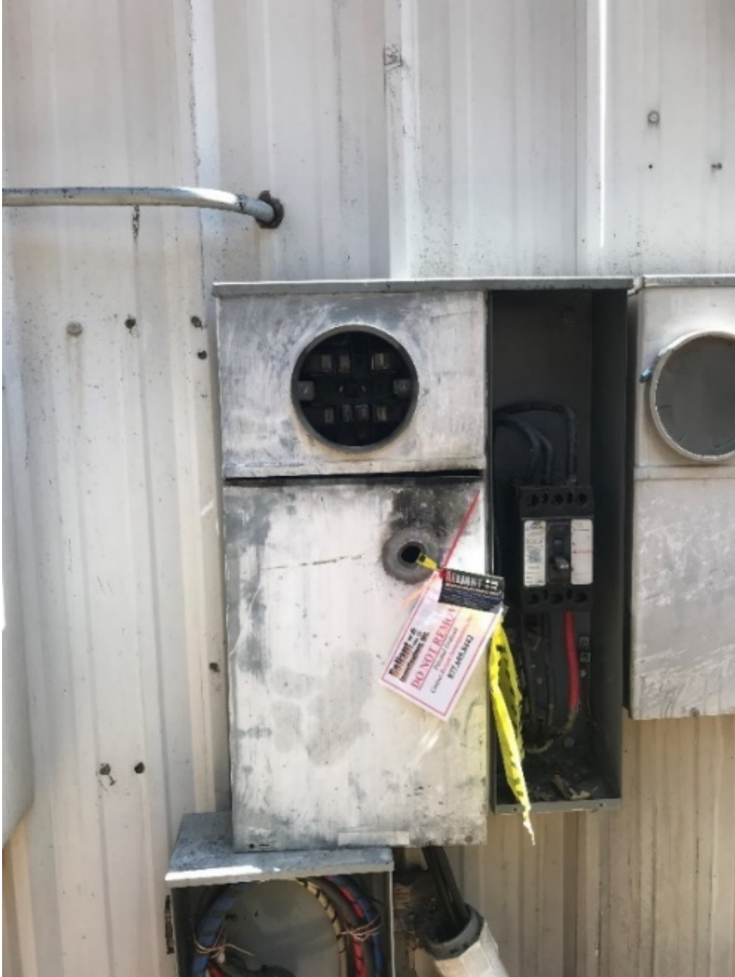
Figure 3: Customer panel. Photo taken during site visit on July 19, 2021.
