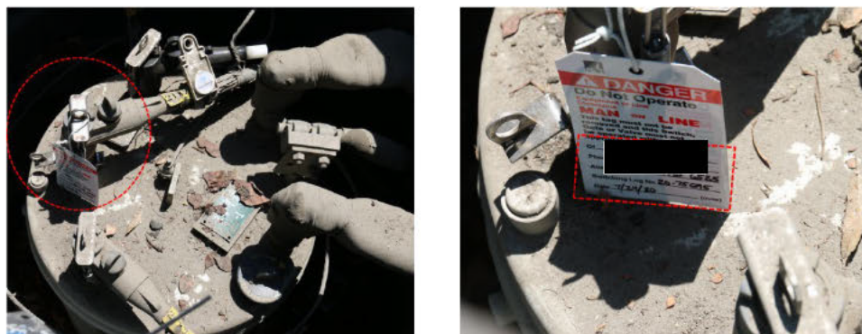
Figure 7: The primary cable toward switch 6525 at the transformer T2142 is lifted and tagged out. Photo taken on August 4, 2020.
