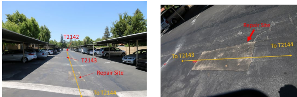
Figure 4: Repair site between transformers T2143 and T2144 on the southeast driveway of the [REDACTED]. The area was repaired on or after July 22 and before July 24, 2020. Photo taken on August 4, 2020.
