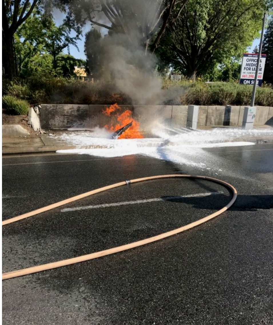
Figure 9: Fire at the underground vault housing the 3-way switch. Photo taken on July 25, 2020.
