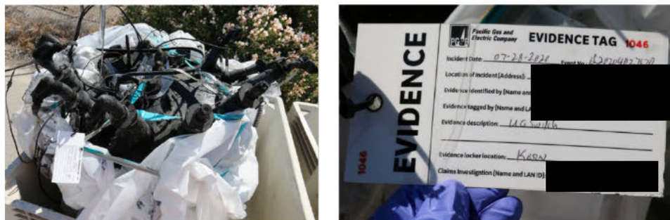
Figure 11: The failed 3-way switch (11003, 11004, 11005) kept in evidence locker. Photo taken on August 4, 2020.
