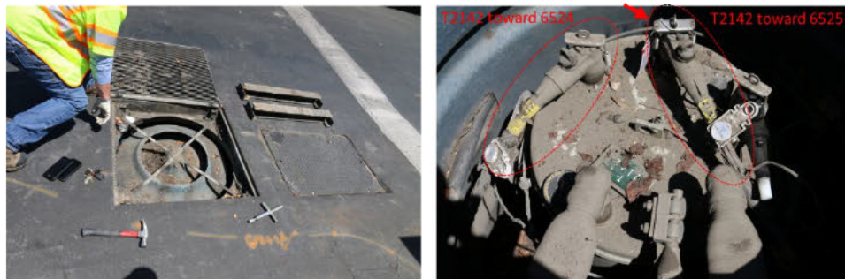
Figure 6: T2142 transformer location. Photo taken on August 4, 2020.
