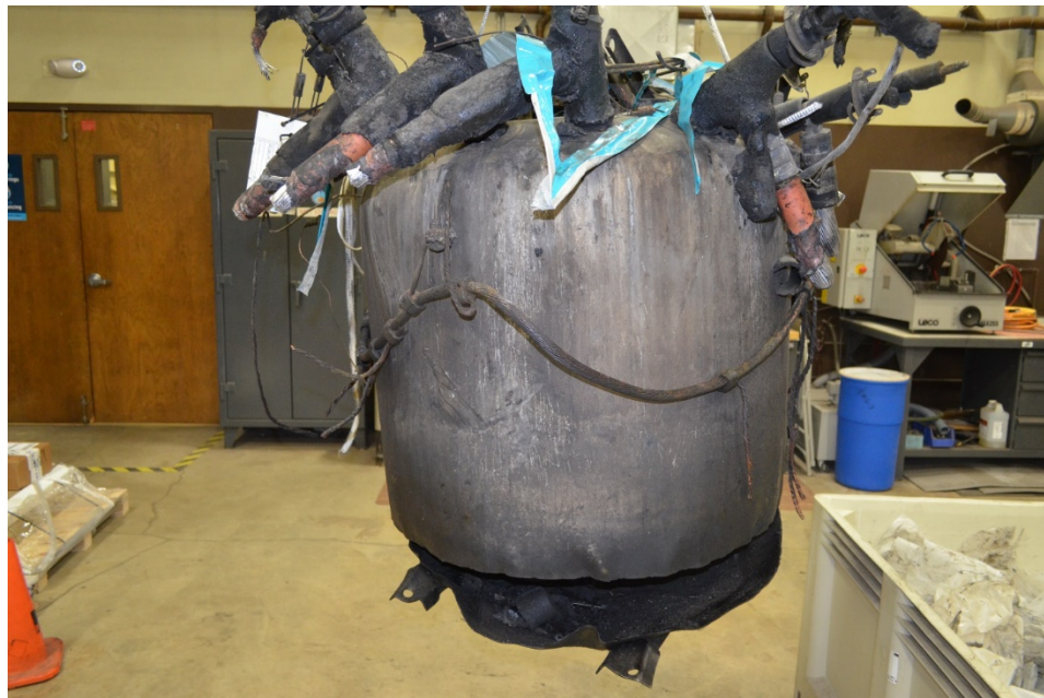
Figure 12: The failed 3-way switch in PG&E's Applied Technology Services Facility in San Ramon, CA. Photo taken on October 7, 2020.
