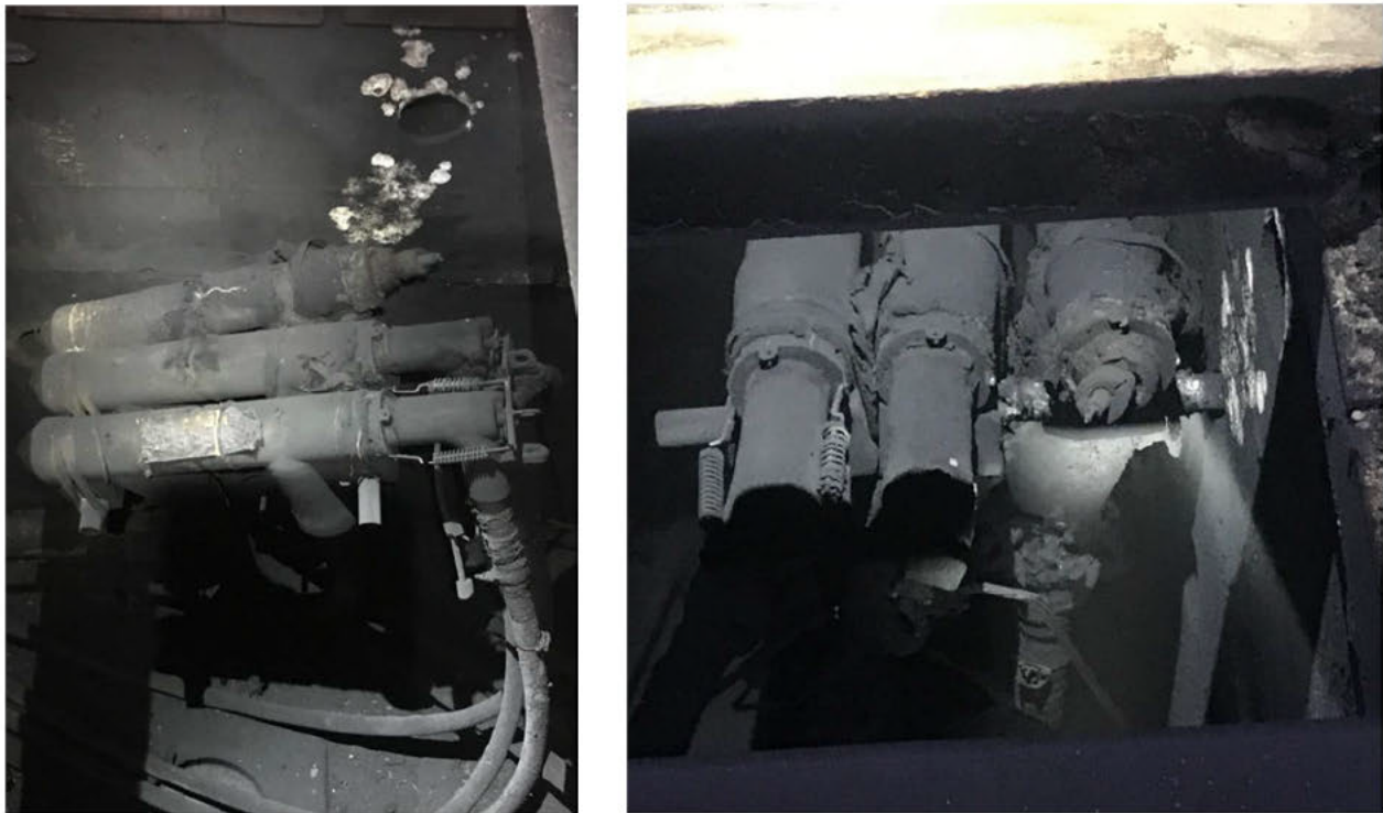
Figure 2: Condition of the damaged equipment on the night of the incident.
