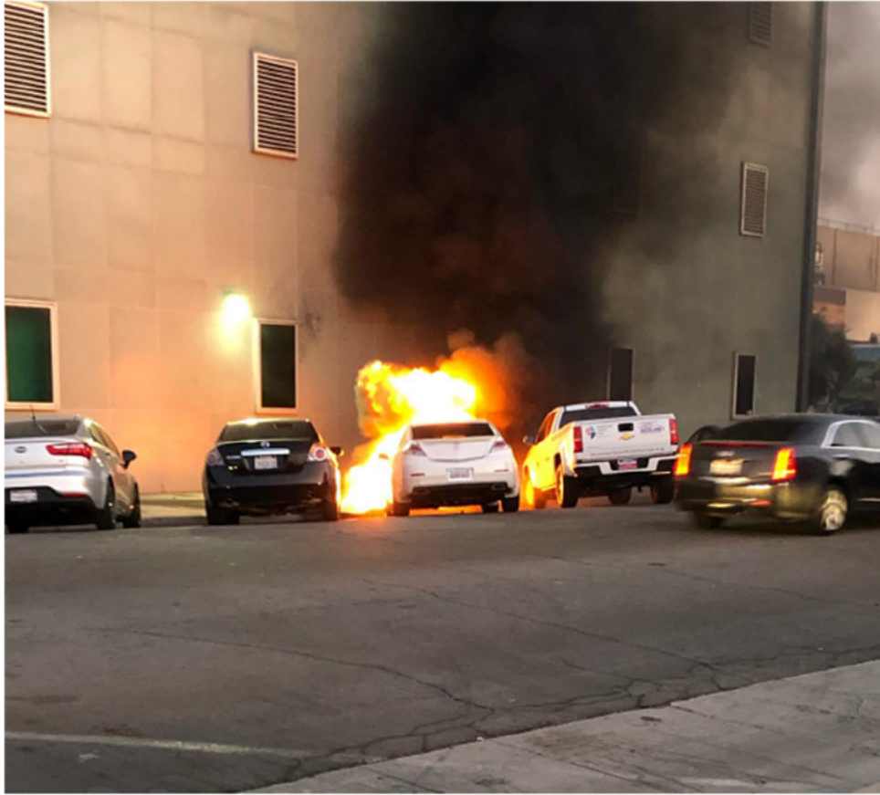
Figure 1: Fire in Vault 39, 20 th and Eye Street, Bakersfield, 11/20/2018. Source: Media
