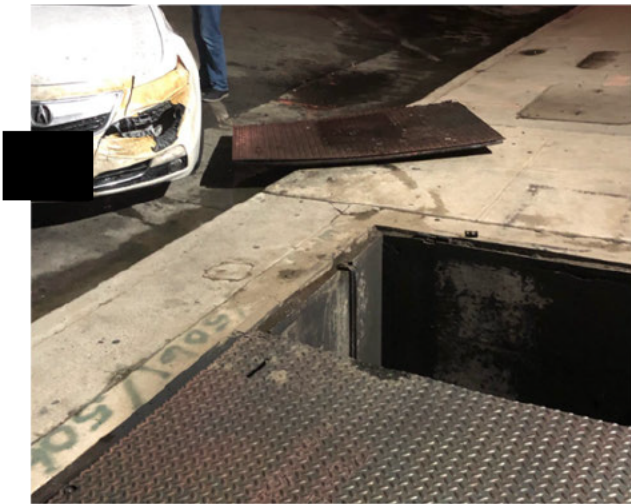
Figure 2: Vault 39 lid and damaged vehicle, 20 th and Eye Street, Bakersfield, 11/20/2018. Source: PG&E
