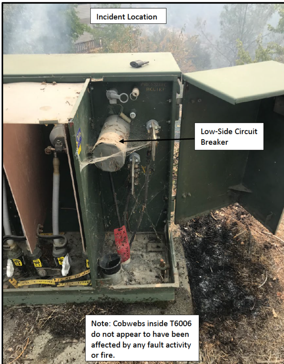
Figure 5: 09/09/20 PG&E troubleshooter image obtained post-incident of Transformer T6006
