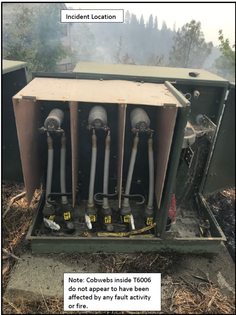
Figure 4: 09/09/20 PG&E troubleshooter image obtained post-incident of Transformer T6006
