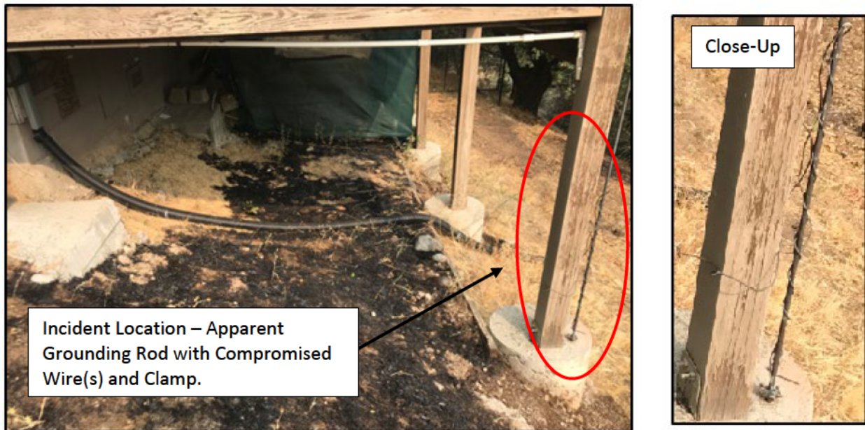
Figure 11: 09/09/22 PG&E troubleshooter Image – Apparent Grounding Rod with Possible Broken Wire - Incident Location
