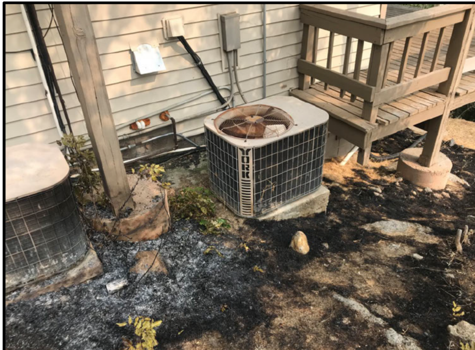
Figure 7: 09/09/22 PG&E troubleshooter image obtained post-incident of AC units at Incident Location
