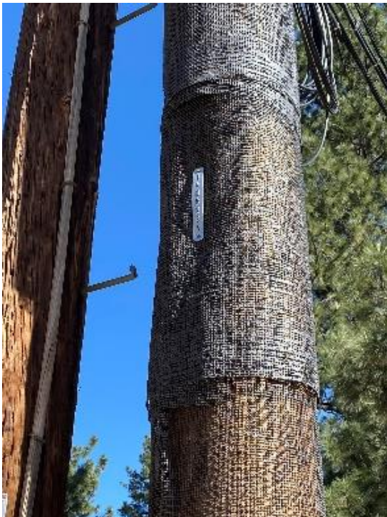
BVES Wooden Pole #14028BV; photo provided by BVES
