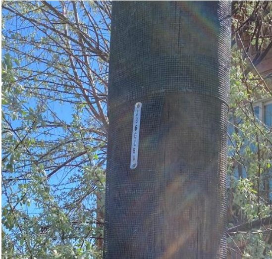
BVES Wooden Pole #13661BV; photo provided by BVES
