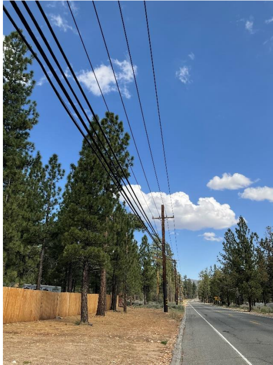
Figure 2-9 — Representative Photo of Installed Covered Conductor
