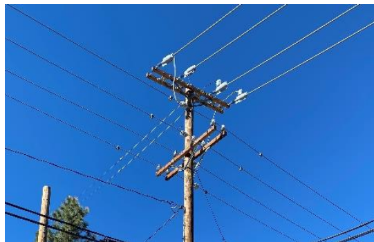
BVES Wooden Pole #14028BV Showing Installed Fault Indicators from two directions; photo provided by BVES
