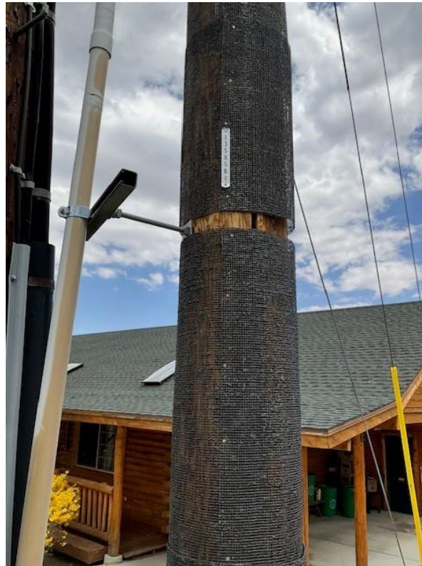
Figure 2-20 — BVES Wooden Pole #13585BV Showing Gap in Fire Wrap
