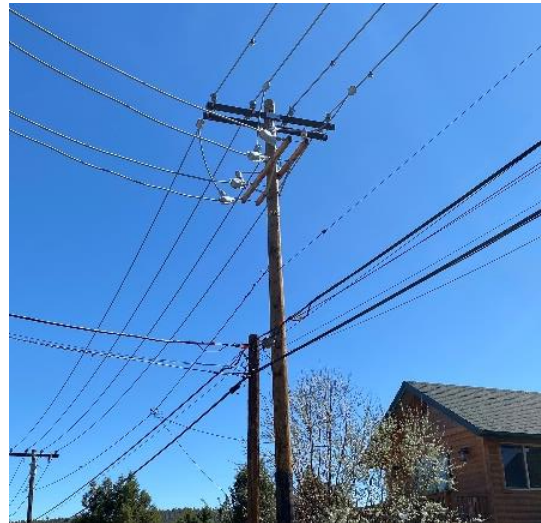
BVES Wooden Pole #13661BV Showing Installed Fault Indicators; photo provided by BVES
