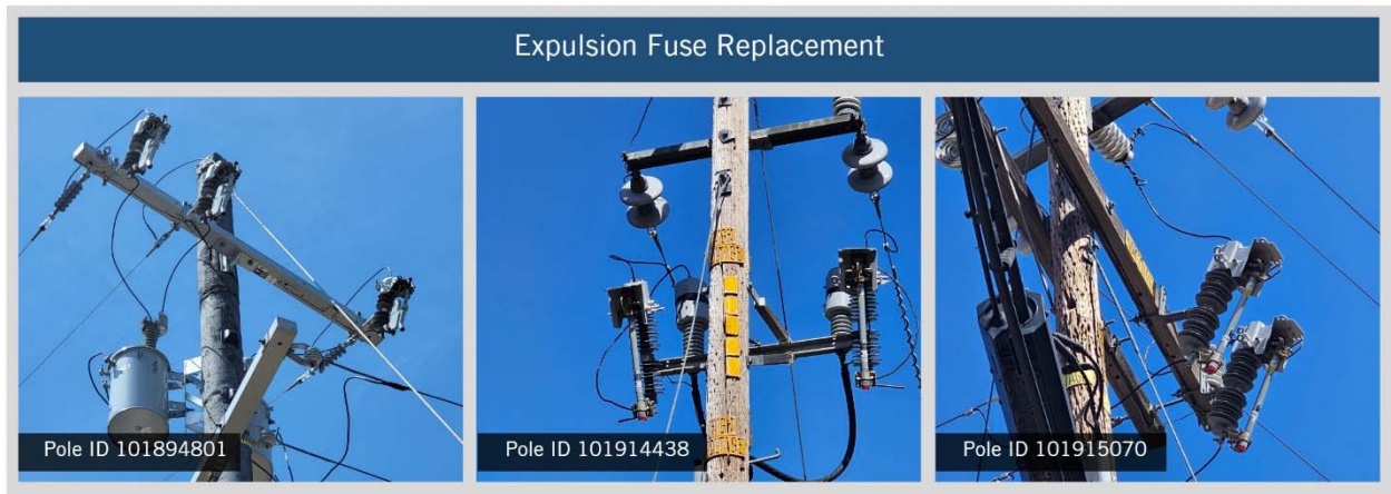
Figure 7: Example Expulsion Fuse Replacement Field Images
