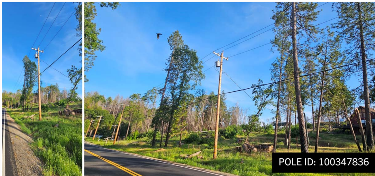
Figure 26: Example Utility Defensible Space with Vegetation Growth Field Image
