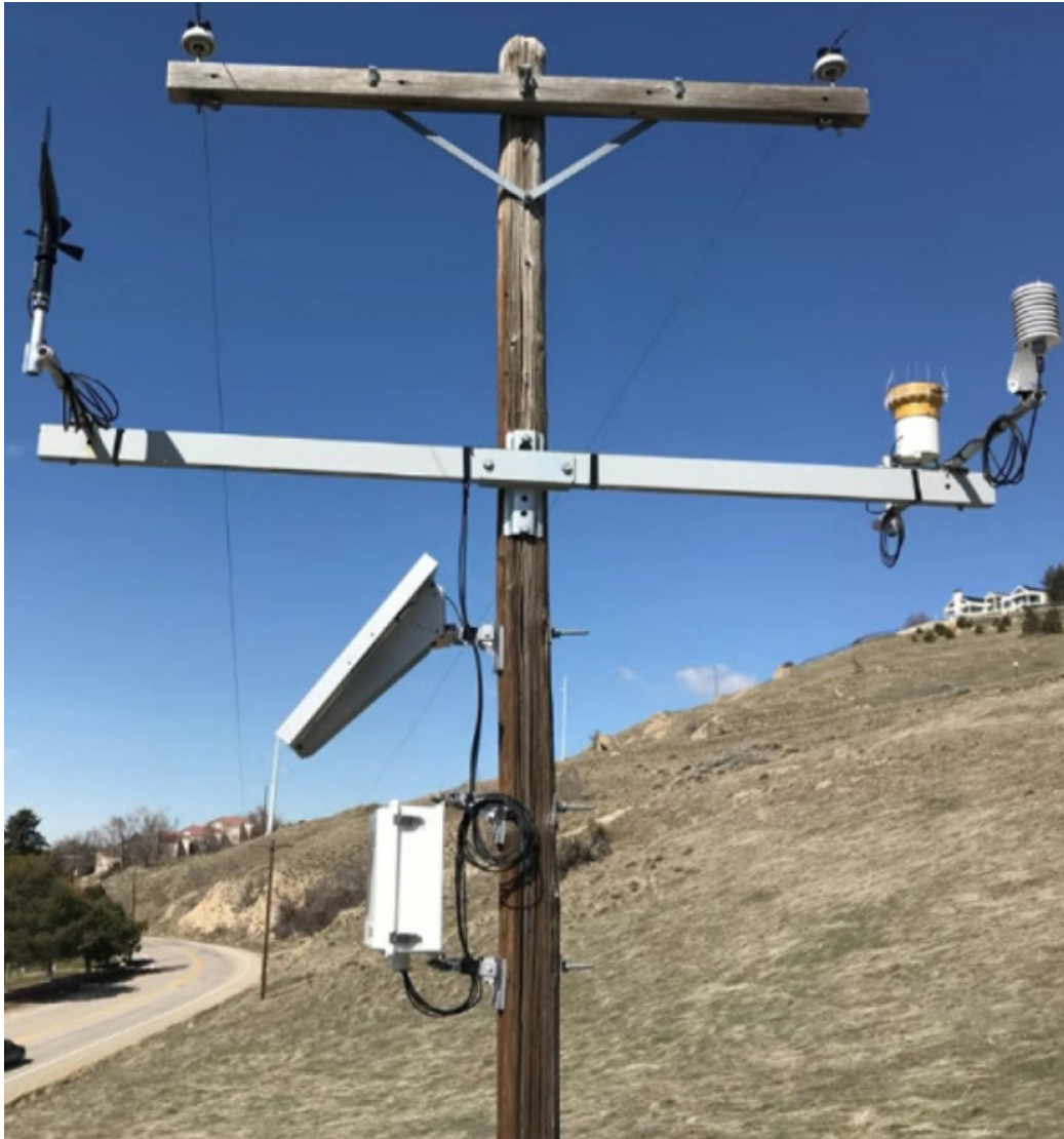
Figure 2—Typical Weather Station Installation on Equipment Arm
