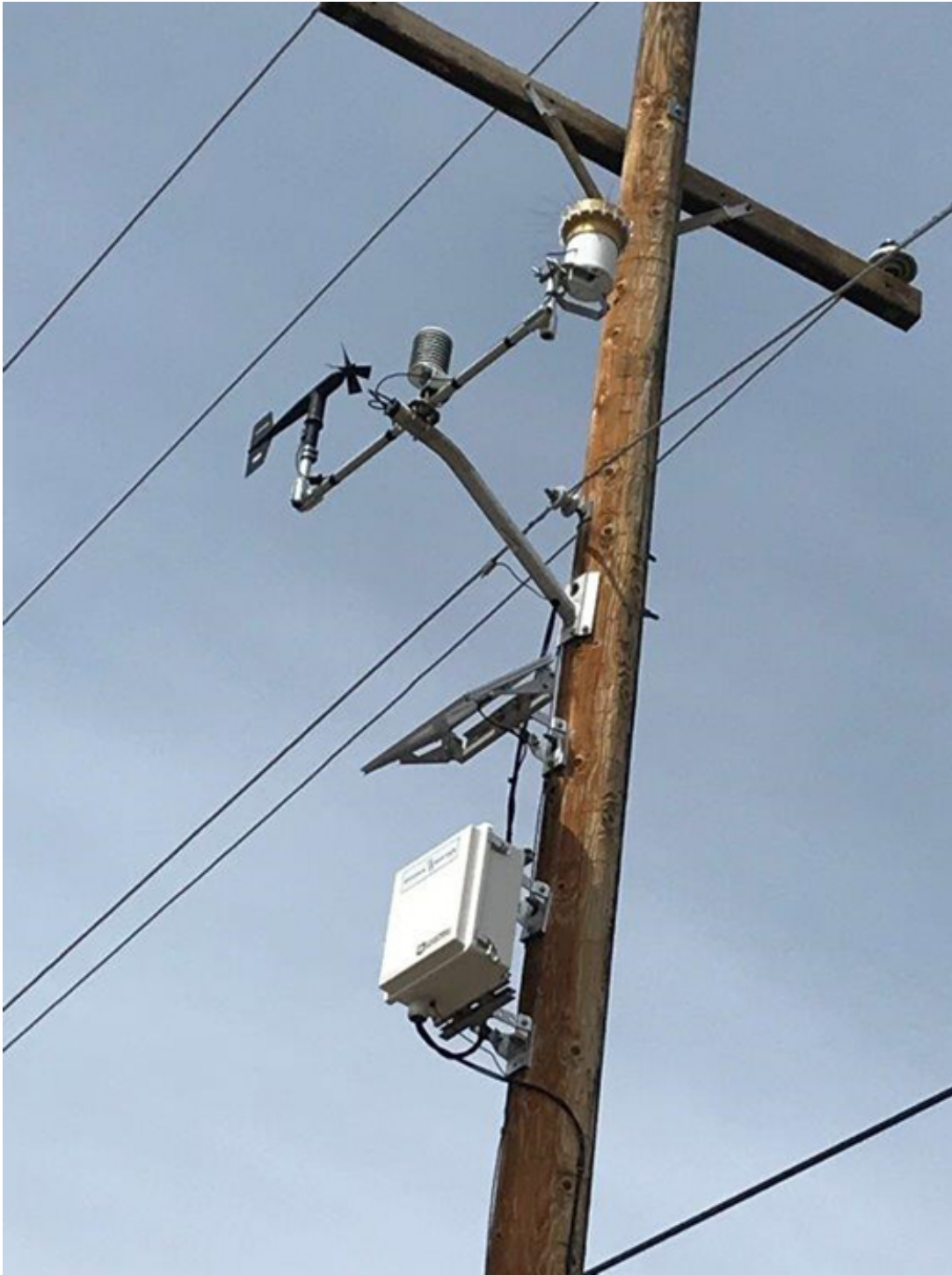
Figure 1—Typical Weather Station Installation on Mast Arm
