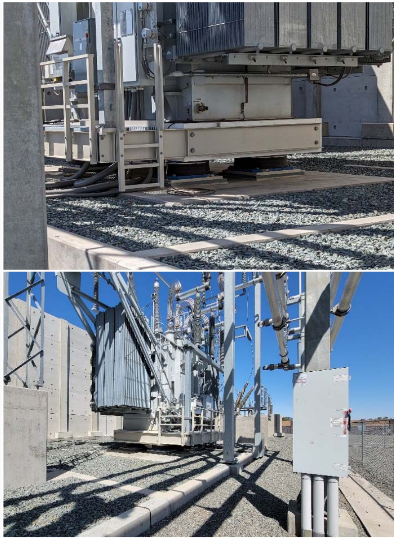
Figure 3: Transformer Seismic Base Isolators and Flame-Suppressing Stone
