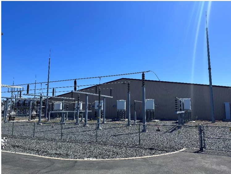
Appendix Figure 4: 180-kV Yard
