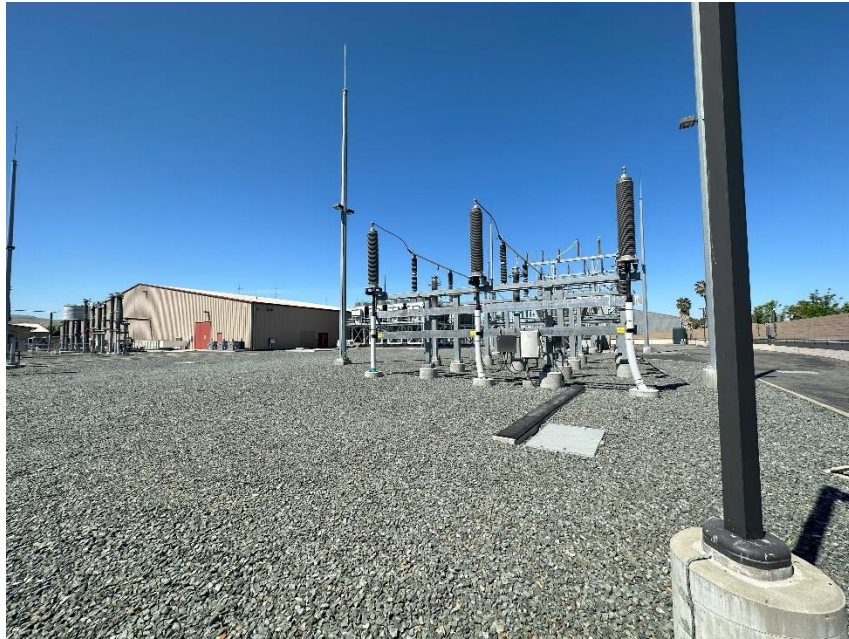
Appendix Figure 6: 230-kV Risers and Circuit Breakers
