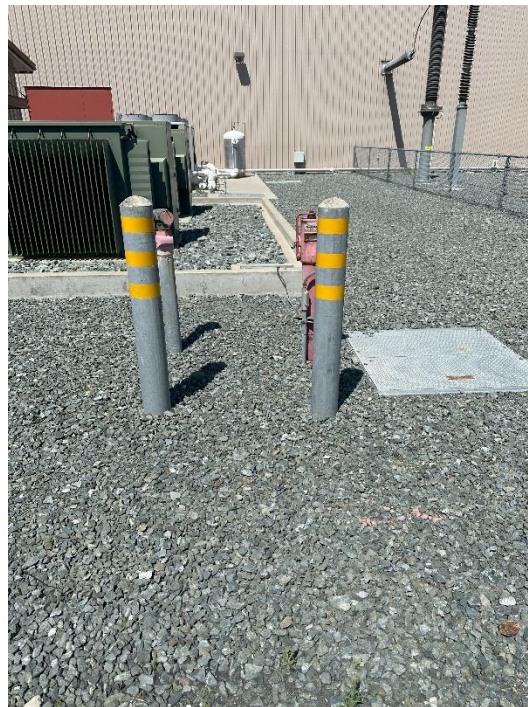
Appendix Figure 7: 200-kV DC Yard
