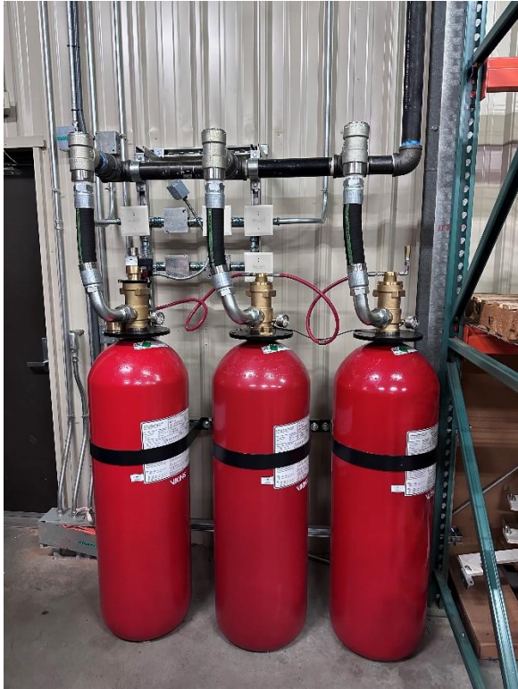
Figure 13: Clean Agent System Tanks
