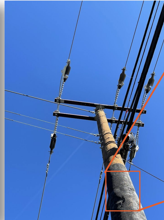
Image source: Green Grid Inc – Fire retardant material at the base of a distribution pole
