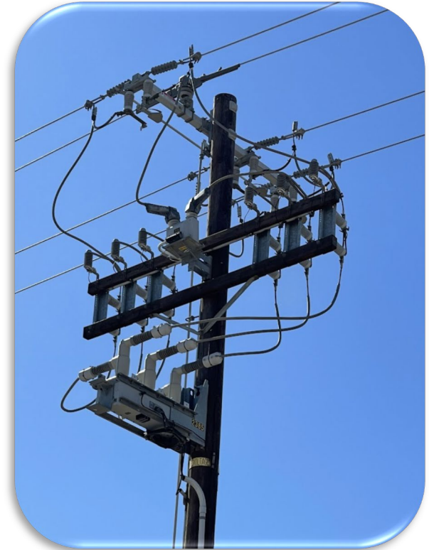
Image source: Green Grid Inc. - Remote activated recloser on composite pole
