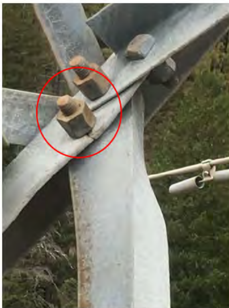
Condition: 4 Priority: E+
