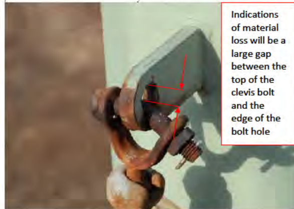
Condition: 4 Priority: E+ FDA (1): Hardware-Tower|No Good/ Out of Std |Replace FDA (2): Insulator-Steel|No Good/ Out of Std |Replace
