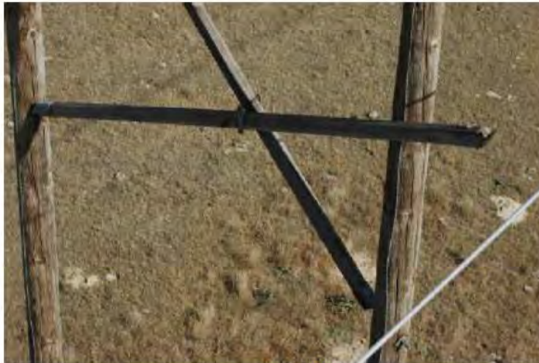
Figure 61 Failed H-frame crossarm (left). Failed crossarm bracing (right).
