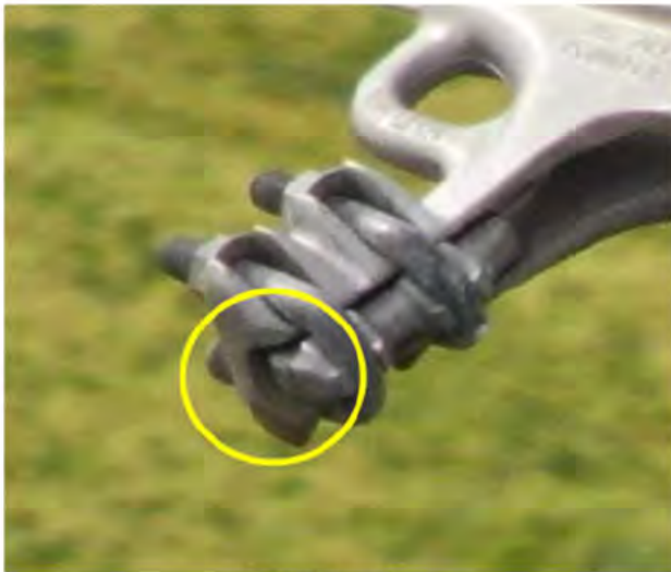
Condition: 5 Priority: A FDA: Emergency | Storm-related | Repair
