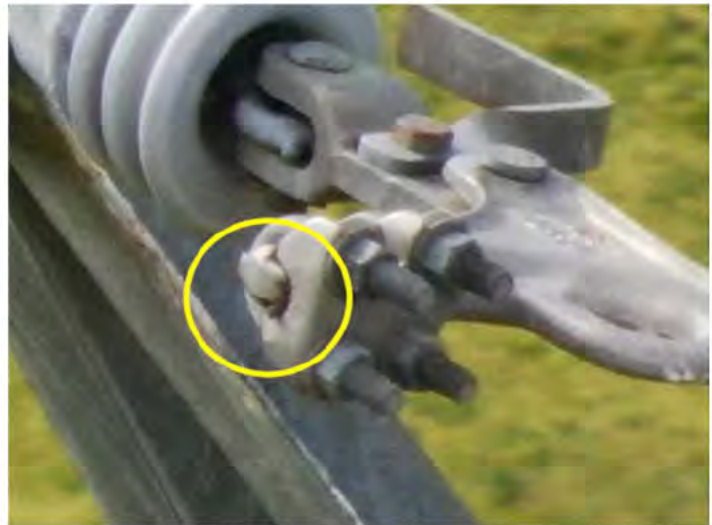
Condition: 4 Priority: E+ FDA: Shield Wire/ OPGW-Steel | No Good/Out of Stdrd | Repair
