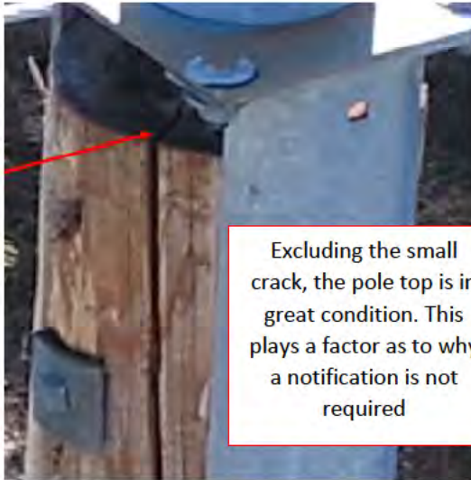
Figure 49 Wide pole crack penetrating roughly 50% of the pole (left). Single small woodpecker hole (right).
