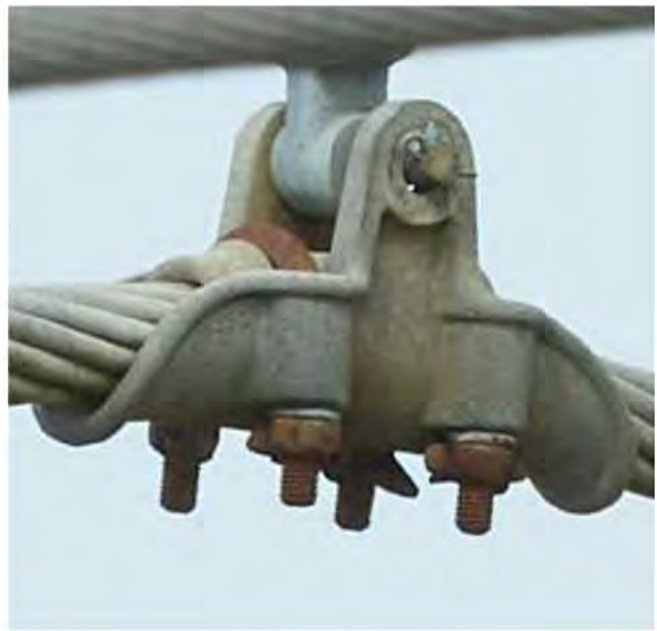
Condition: 3 Priority: E
