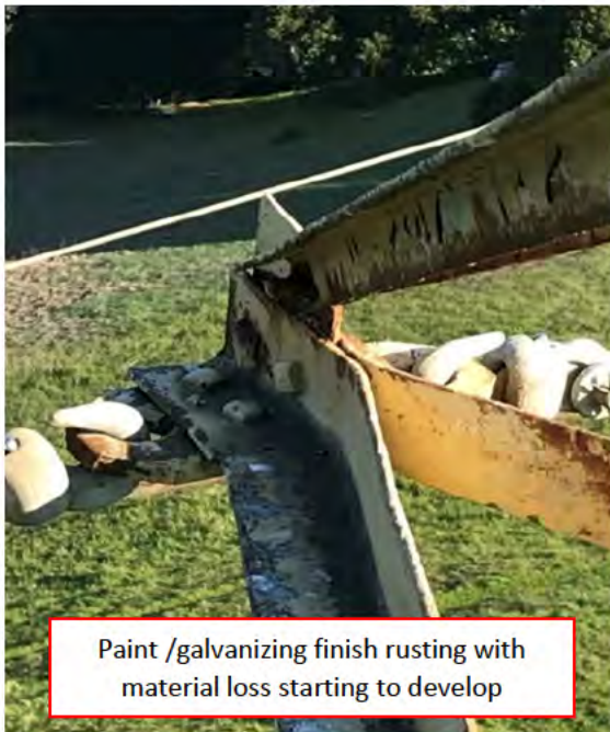
Critical/main member corrosion with 30-50% material loss (left). Old tower foundation (CIRT to contact civil engineering for action) (right).
