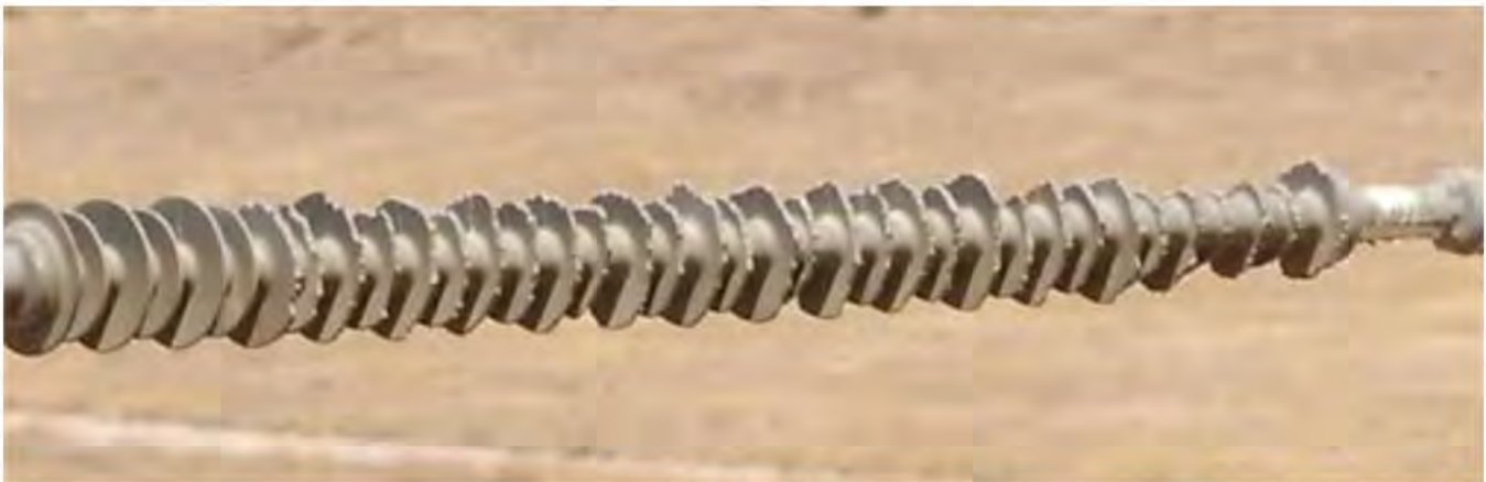
Figure 128 Flashed polymer insulator (left). Minor damage to polymer sheds (right).
