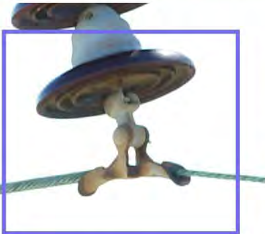
Figure 139 Broken pin insulator biscuit at connection hardware.
