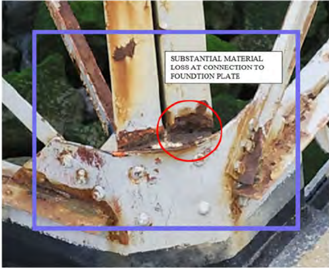
Condition 4 Priority E+
