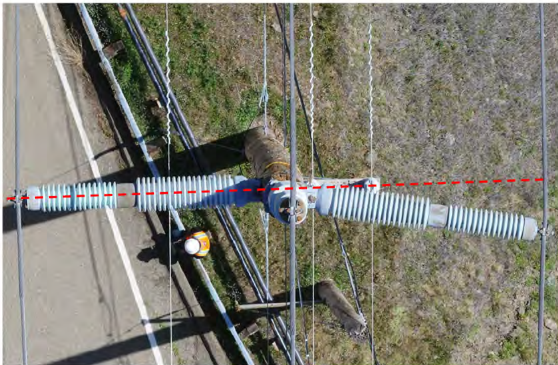
Figure 112 Out of plumb insulators. Insulators extremely out of plumb require replacement, rather than repair.
