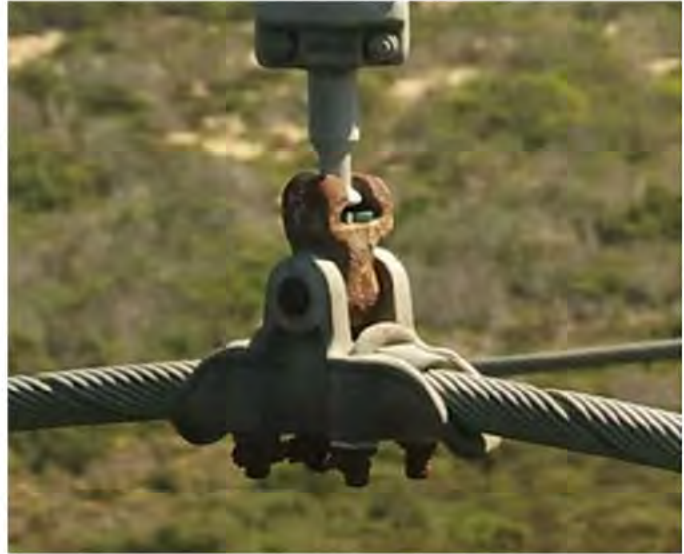
Condition: 3 Priority: E FDA: Insulator-Wood/Steel|No Good/ Out of Stdrd |Repair
