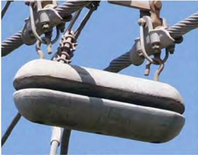
Condition: 3 Priority: E
