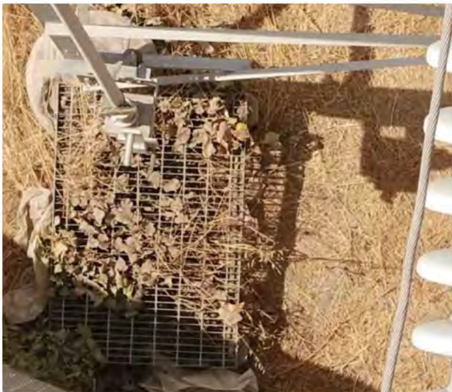
Figure 236 Examples of exposed switch control wiring at ground level.
