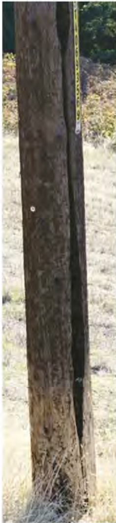
Condition: 4 Priority: E+ FDA: Structure-Wood|No Good/ Out of Stdrd | Replace
