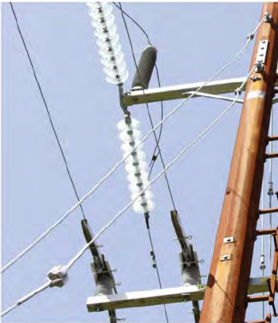
Figure 28 Loose guy (left). Loose span guy (right).
