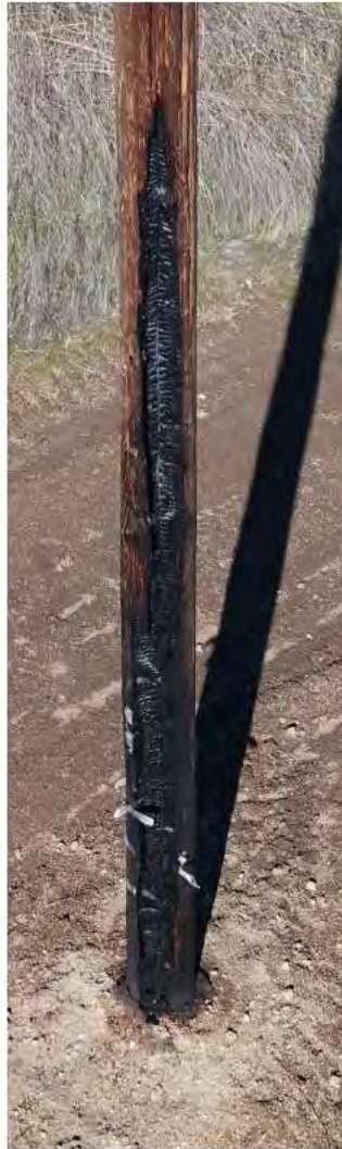
Condition: 4 Priority: E+ FDA: Structure-Wood|No Good/ Out of Stdrd | Replace
