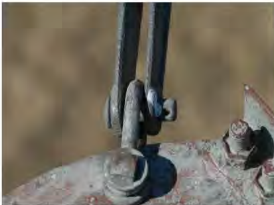
Condition: 4 Priority: E+ FDA: Insulator-Steel|No Good/ Out of Std |Repair
