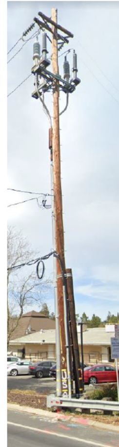
Stubbed Riser Pole on Jefferson-Stanford 60 kV
