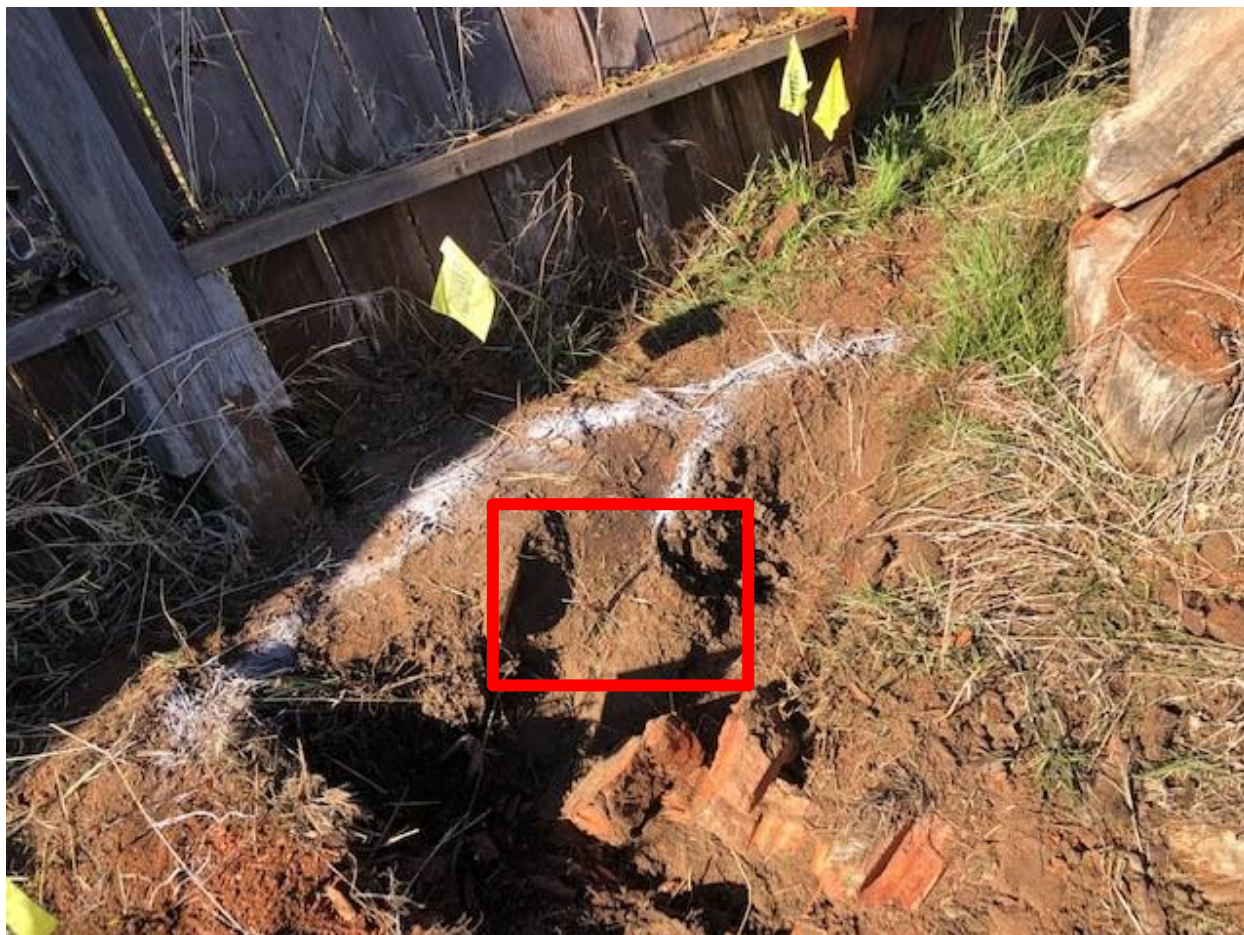
Photo 2: Photo of the damaged facility provided by Sacramento County Regional Parks. Red rectangle indicating the damaged facility added by investigator.
