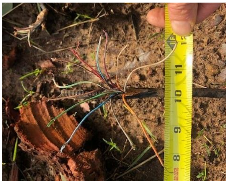
Photo 3: Photo of the diameter of the damaged facility provided by Sacramento County Regional Parks.
