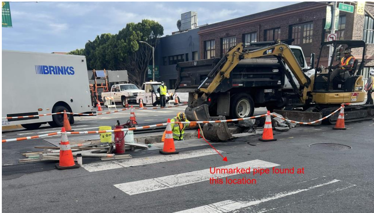
Photo 2: Photo and description in red provided by Phoenix Electric Company.
