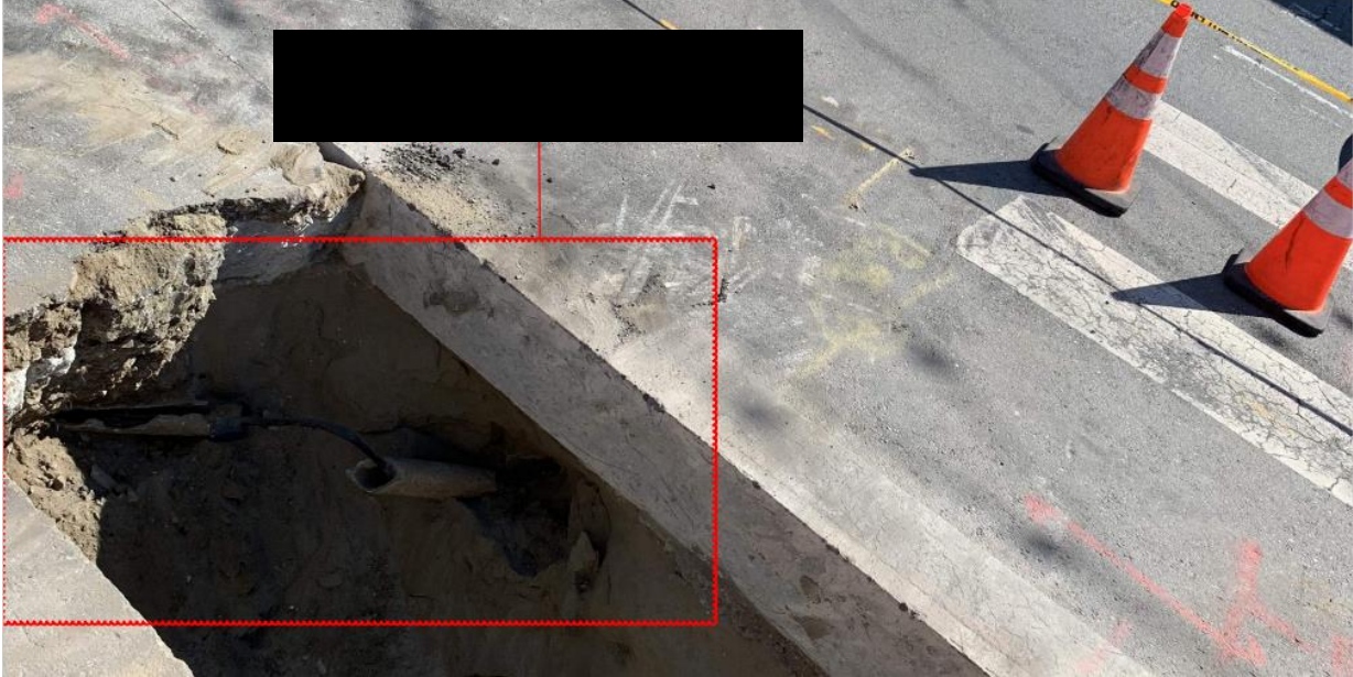
Photo 3: Photo and box in red provided by Phoenix Electric showing the facility conduit and interior cable running roughly north-south along Potrero Street. Black box inserted by investigator to remove uncertain description provided by Phoenix Electric Company.
