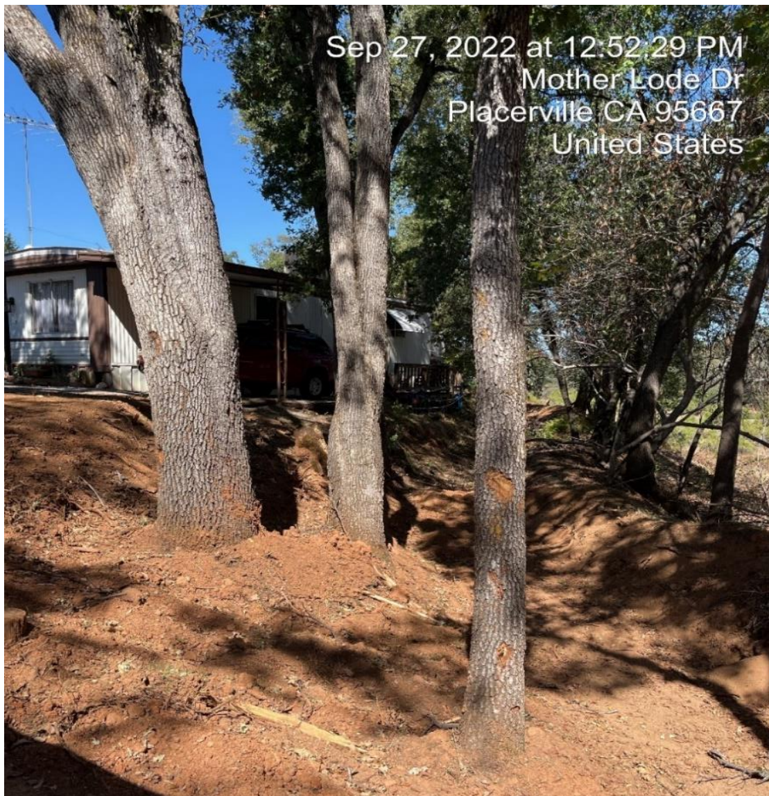
Photo 3: Photo of trenched area adjacent to the pumphouse and Unit 32 located in the background taken by investigator.
