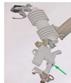
S&C Fault Tamer Fuse - Open
