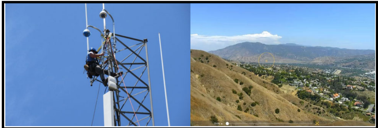
Figure 6: High Resolution Camera Installation and Camera Image Overlooking Anaheim
