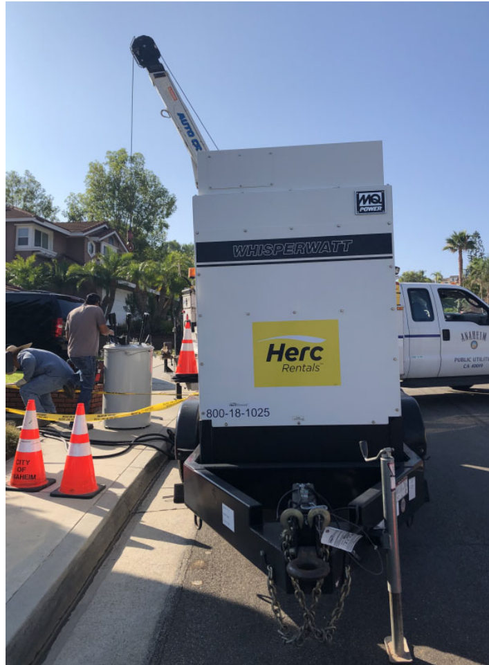
Figure 17: APU Emergency Generator
