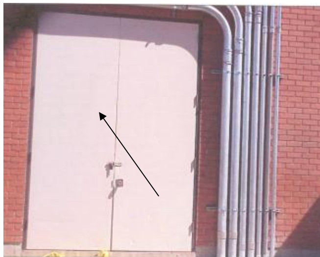
No High Voltage Sign Missing Code 5 (Infraction)
