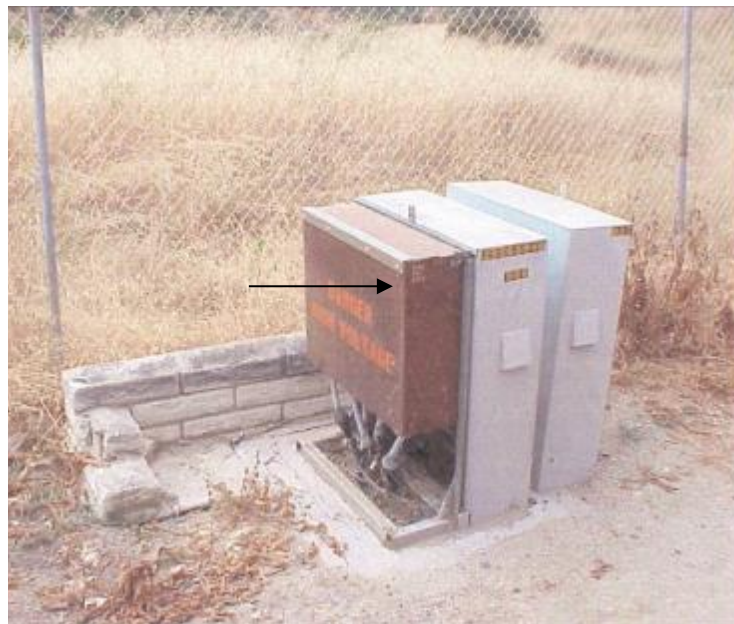
High Voltage Sign Damaged or Missing (Livefront) Code 5 (Infraction)
