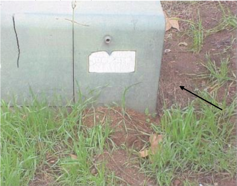
Weeds, Trees, Bushes, Dirt or Obstacle Outside Unit Code 47
