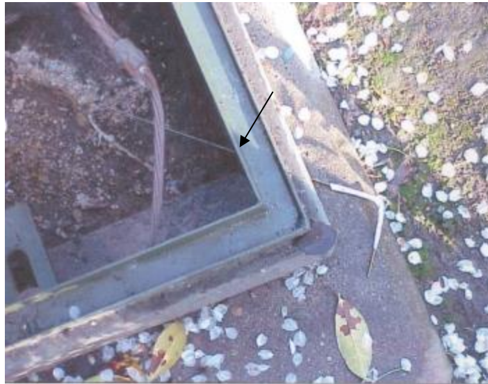
Wire Entry/Severe Corrosion Code 55 – Wire Entry Code 16 – Severe Corrosion
