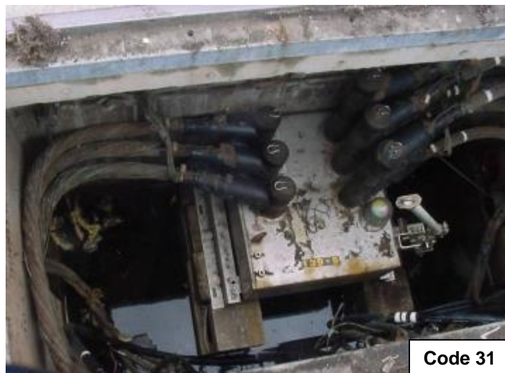
Code 31 (Reliability)- Example of Inadequate Internal Work Space. This is not an infraction because the condition is identified and the structure is tagged "Do Not Enter Energized".
