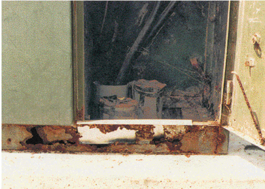
Figure 6-3: Another Example of Metal Flaking Away at Nonhazardous Locations
