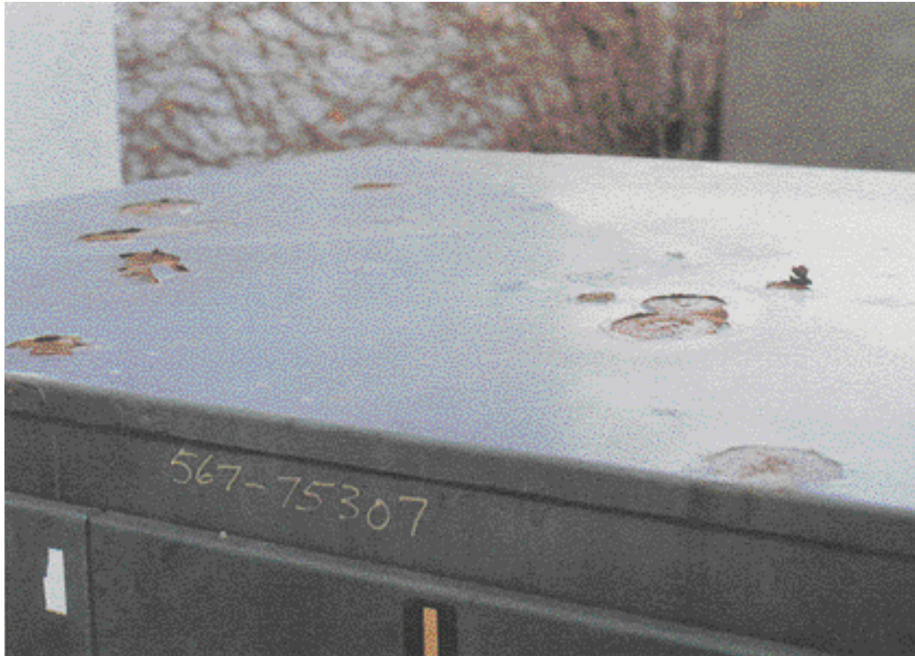
Figure 6-17: Moderate Corrosion with Pitting and Significant Loss of Paint
