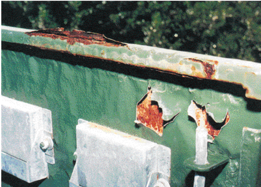
Figure 6–20: Peeling of Paint with Moderate Pitting
