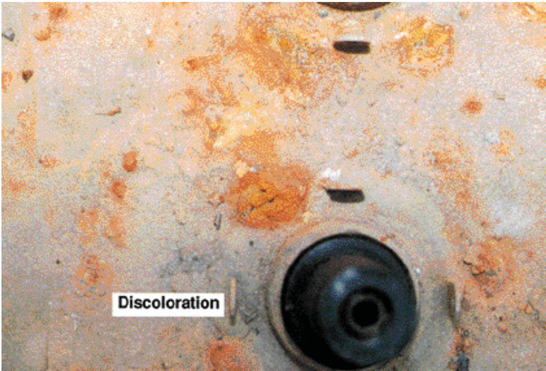
Figure 5–12: Light Corrosion — Example 3 of 3
