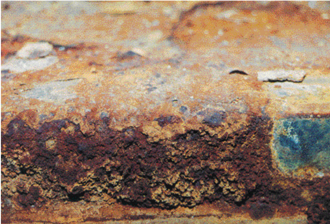
Figure 5–8: Moderate Corrosion — Example 2 of 3
