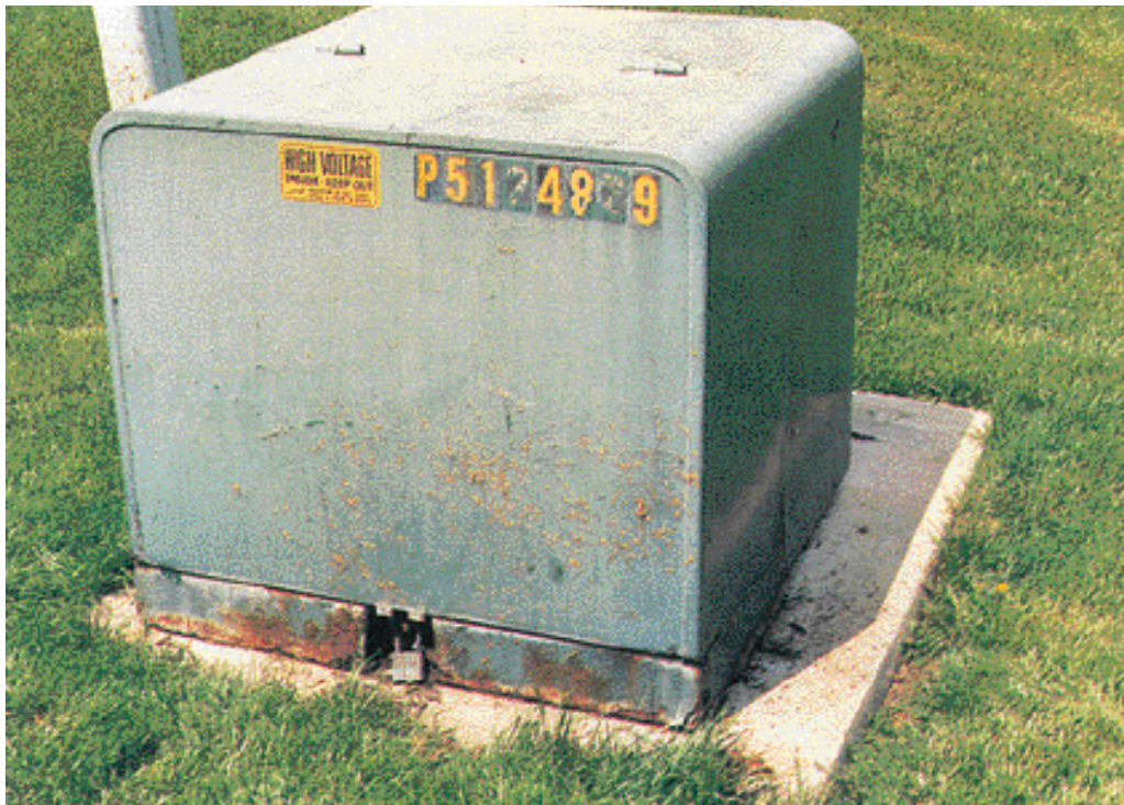
Figure 6-18: Moderate Corrosion with Significant Loss of Paint at Base
