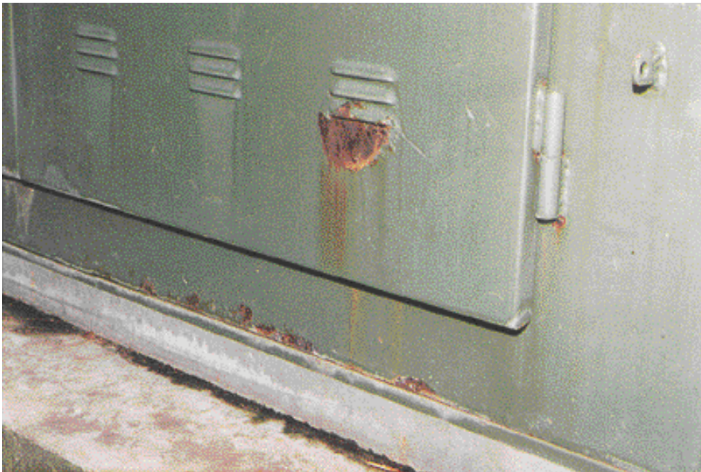
Figure 6–25: Light Corrosion at Louver Openings and at Base of Cabinet (No Serious Pitting)
