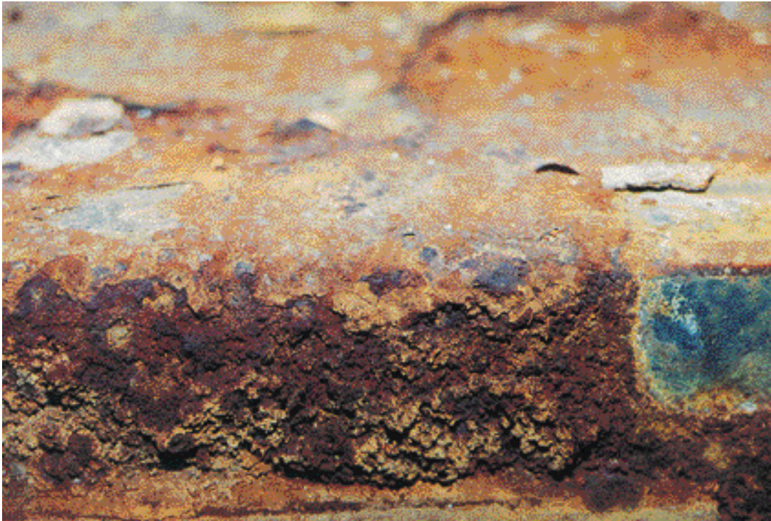
Figure 5–8: Moderate Corrosion — Example 2 of 3
