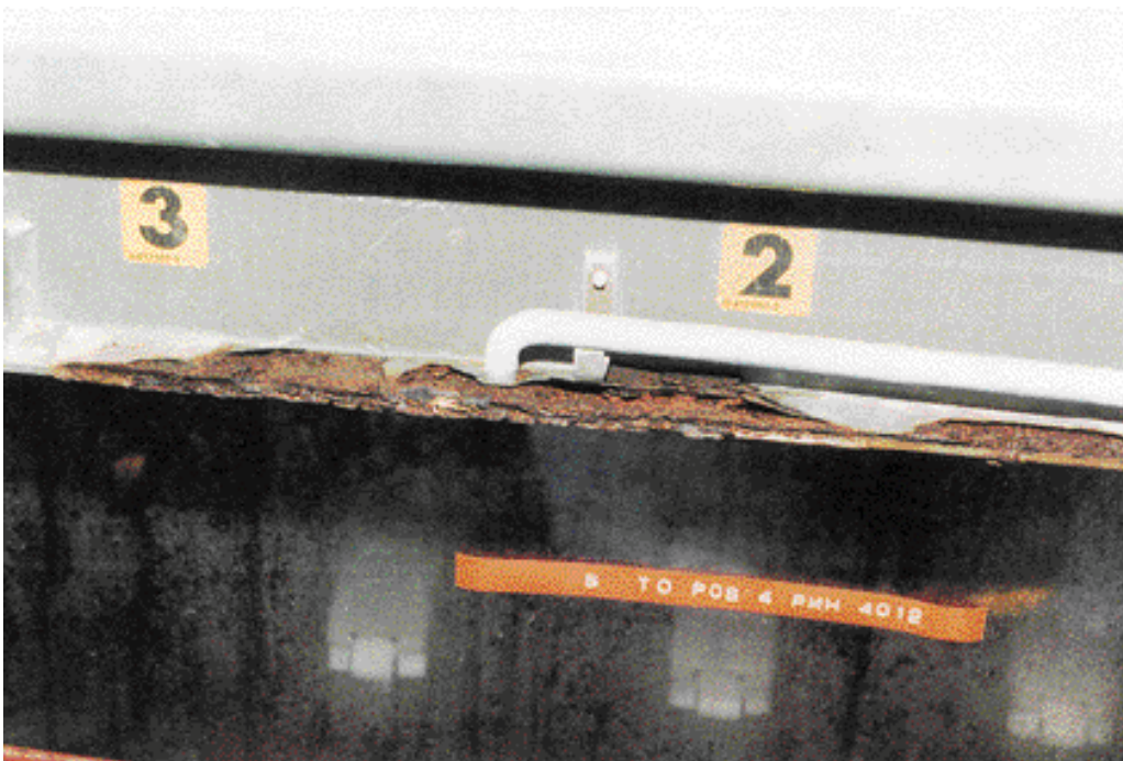
Figure 6–15: Loss of Metal
