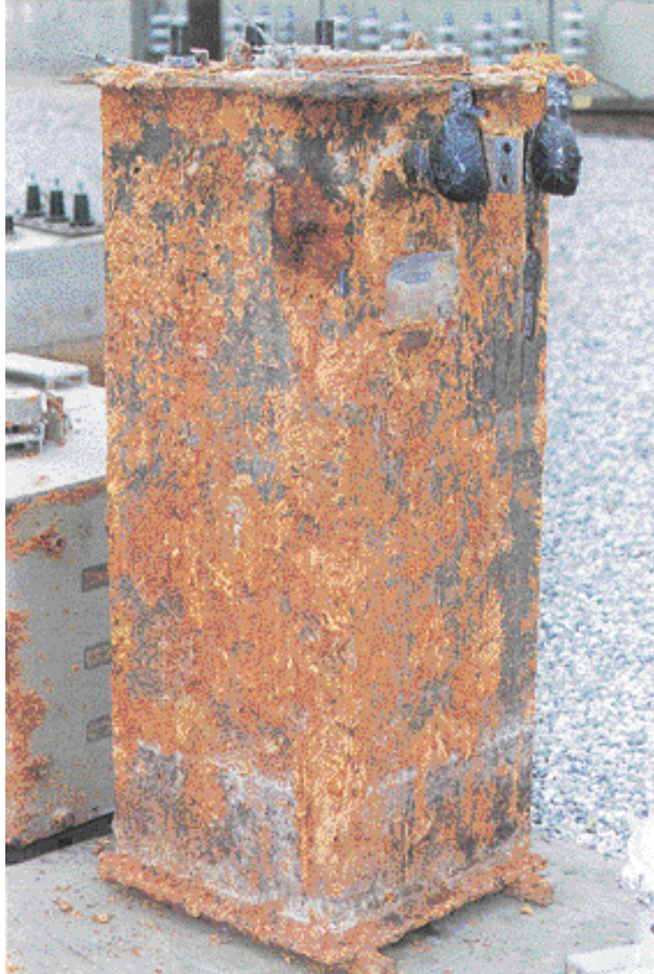
Figure 5-4: Heavy Corrosion — Example 1 of 3
