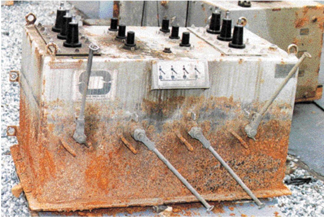
Figure 5-10: Light Corrosion — Example 1 of 3
