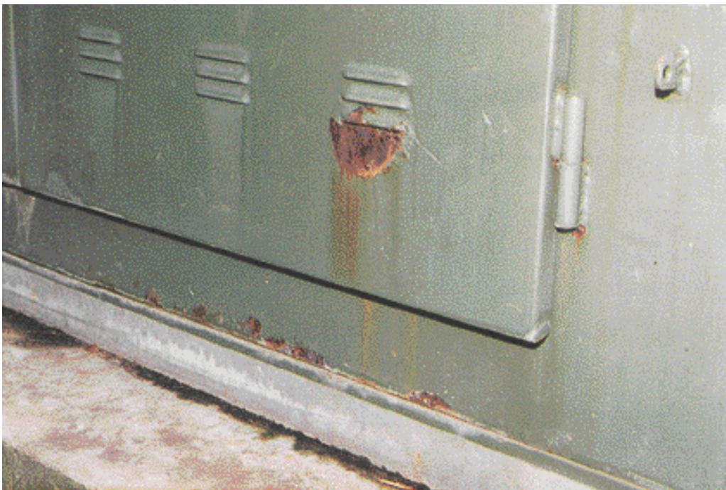
Figure 6–25: Light Corrosion at Louver Openings and at Base of Cabinet (No Serious Pitting)
