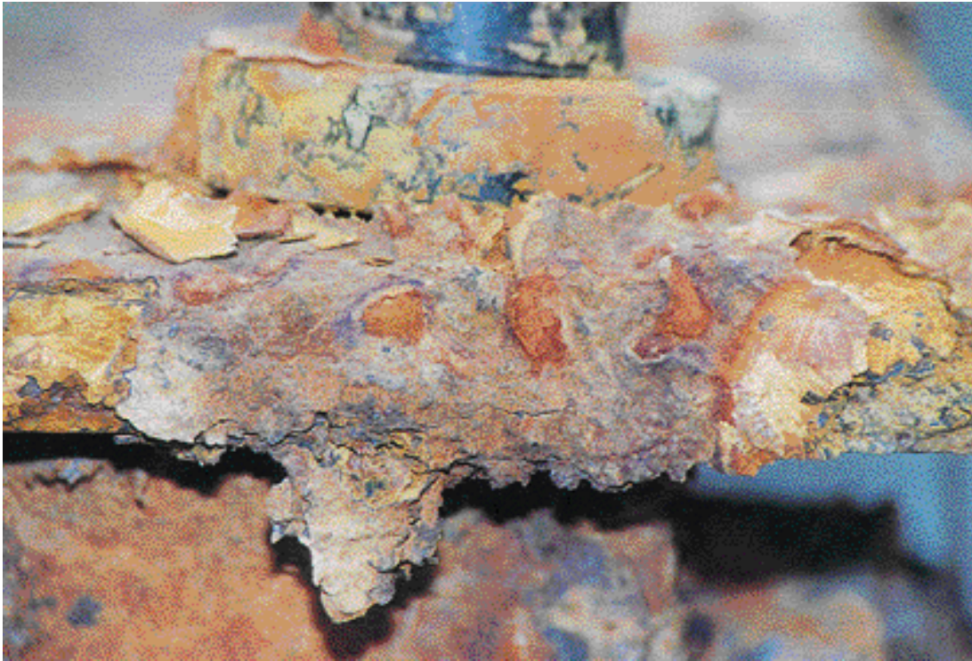
Figure 5-5: Heavy Corrosion — Example 2 of 3
