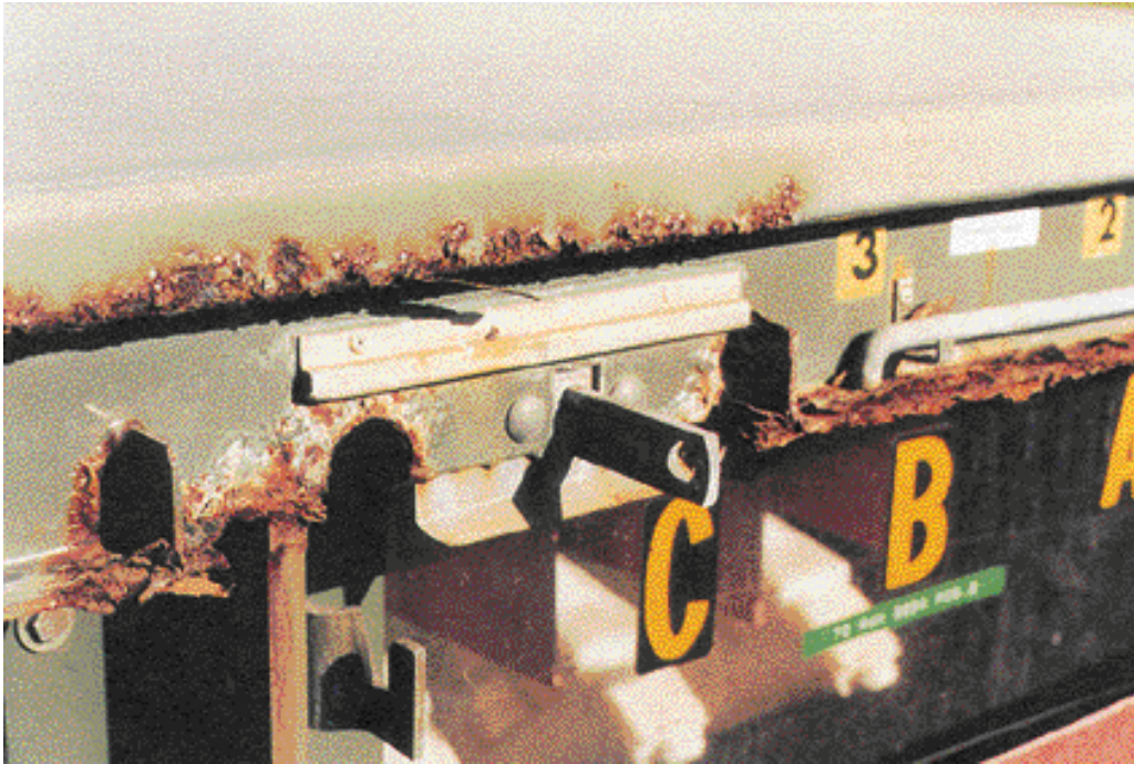
Figure 6–8: Metal Flaking Away at Nonhazardous Locations
