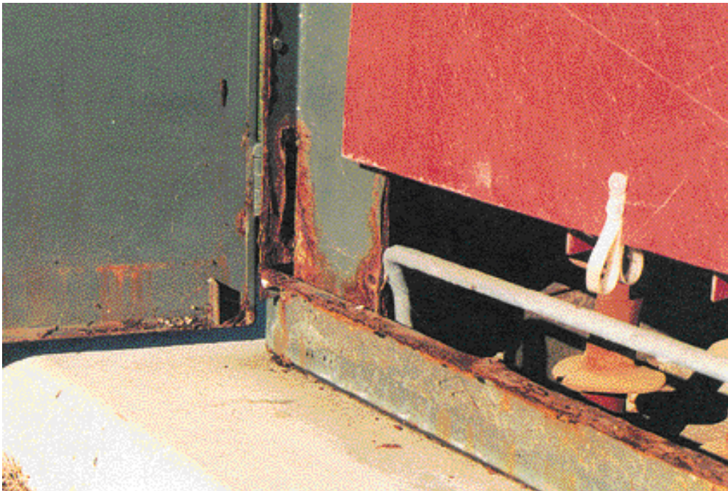
Figure 6–9: Another Example of Metal Flaking Away at Nonhazardous Locations
