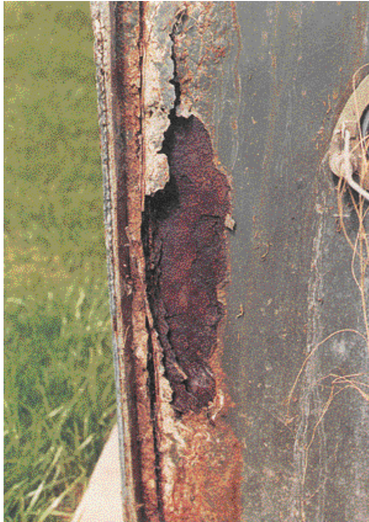
Figure 6–10: Heavy Corrosion with Deep Pitting, Exceeding One-Quarter of Original Wall Thickness
