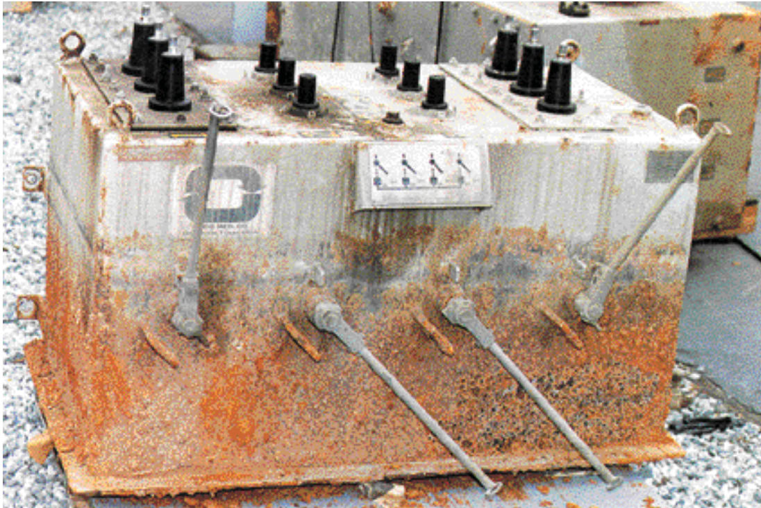
Figure 5-10: Light Corrosion — Example 1 of 3
