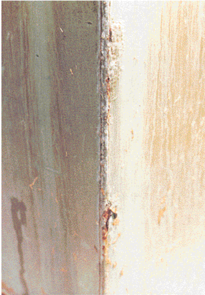
Figure 6–29: Light Corrosion at Weld Seam (No Serious Pitting)
