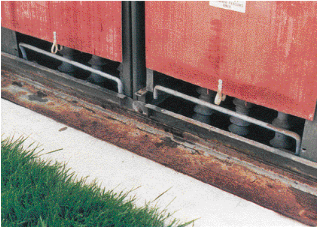
Figure 6-27: Light Corrosion of Adapter Cover Plate (No Serious Pitting)
