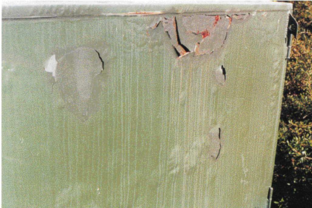
Figure 6–12: Ineffective Prior Repairs
