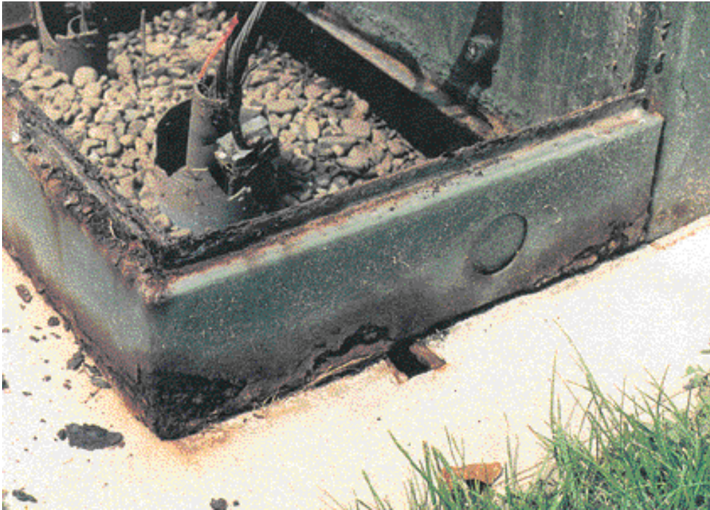
Figure 6–11: Another Example of Heavy Corrosion with Deep Pitting, Exceeding One-Quarter of Original Wall Thickness
