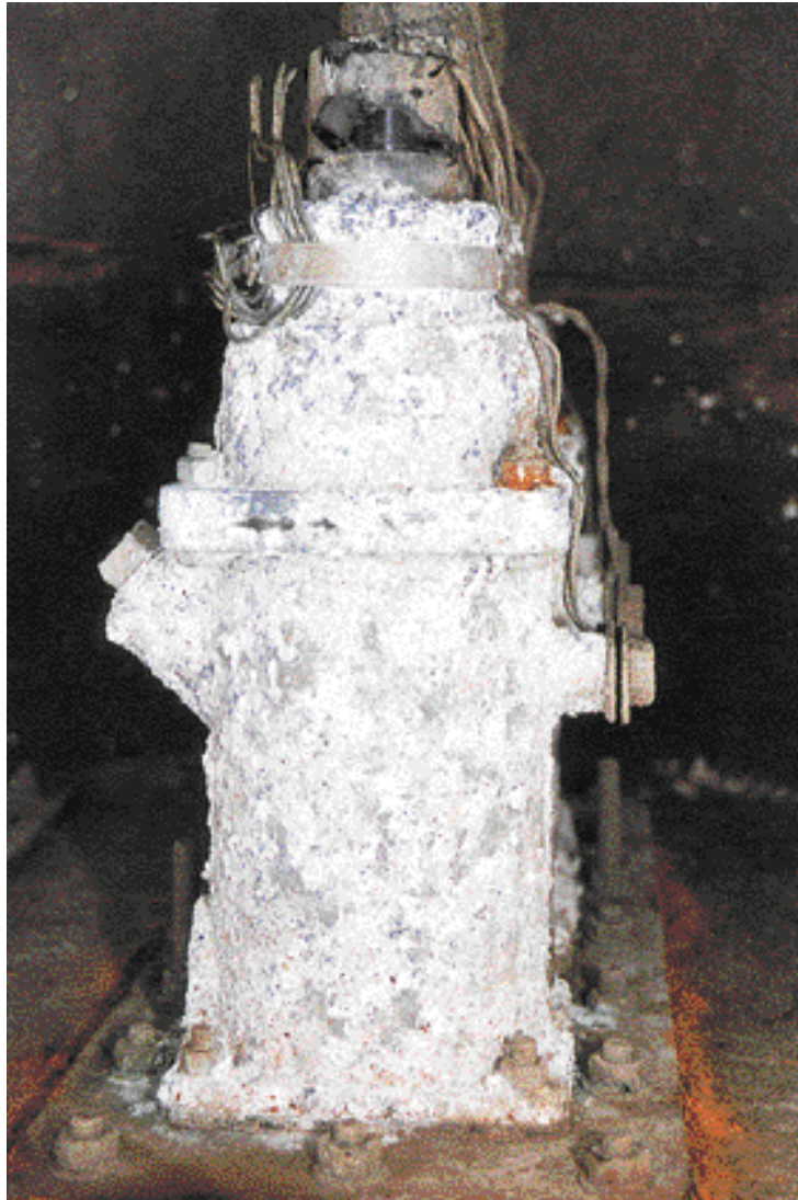
Figure 5–20: Typical Problems — Example 4 of 4
