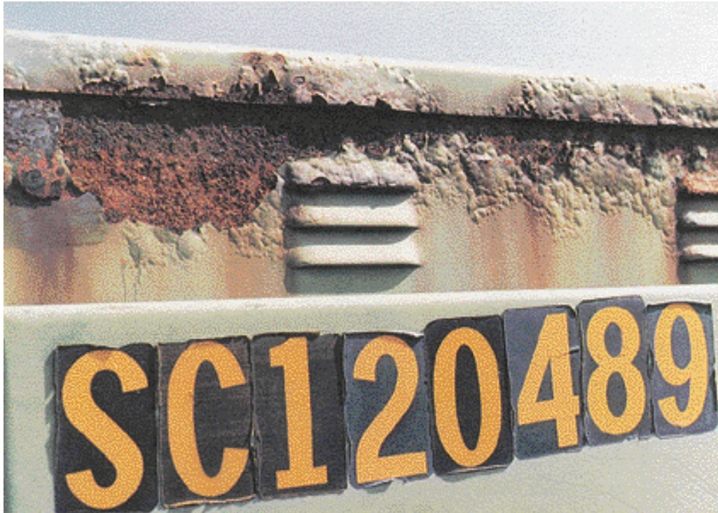
Figure 6-6: Pitting Exceeding One-Quarter Depth of Wall Thickness
