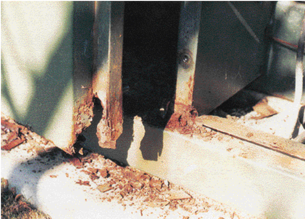
Figure 6-5: Wall Corrosion at Bottom of Compartment Door, Covered when Other Door Closed
