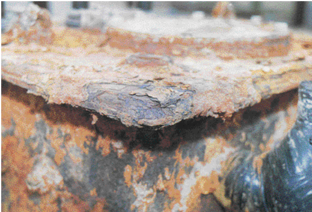
Figure 5-6: Heavy Corrosion — Example 3 of 3
