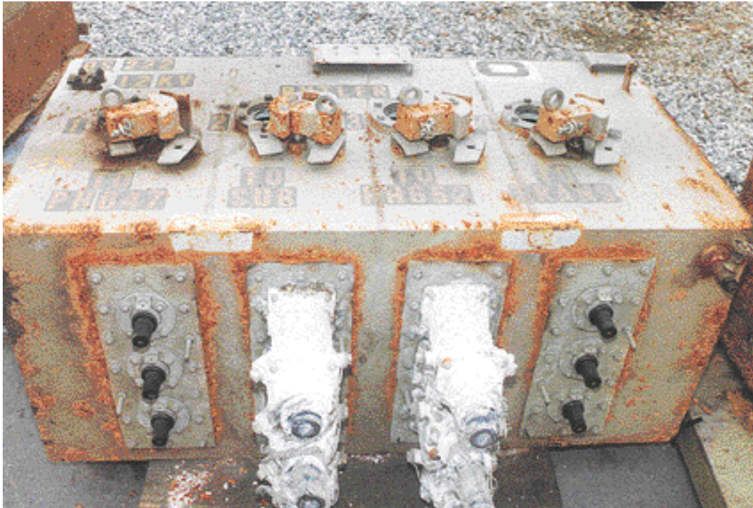
Figure 5–19: Typical Problems — Example 3 of 4
