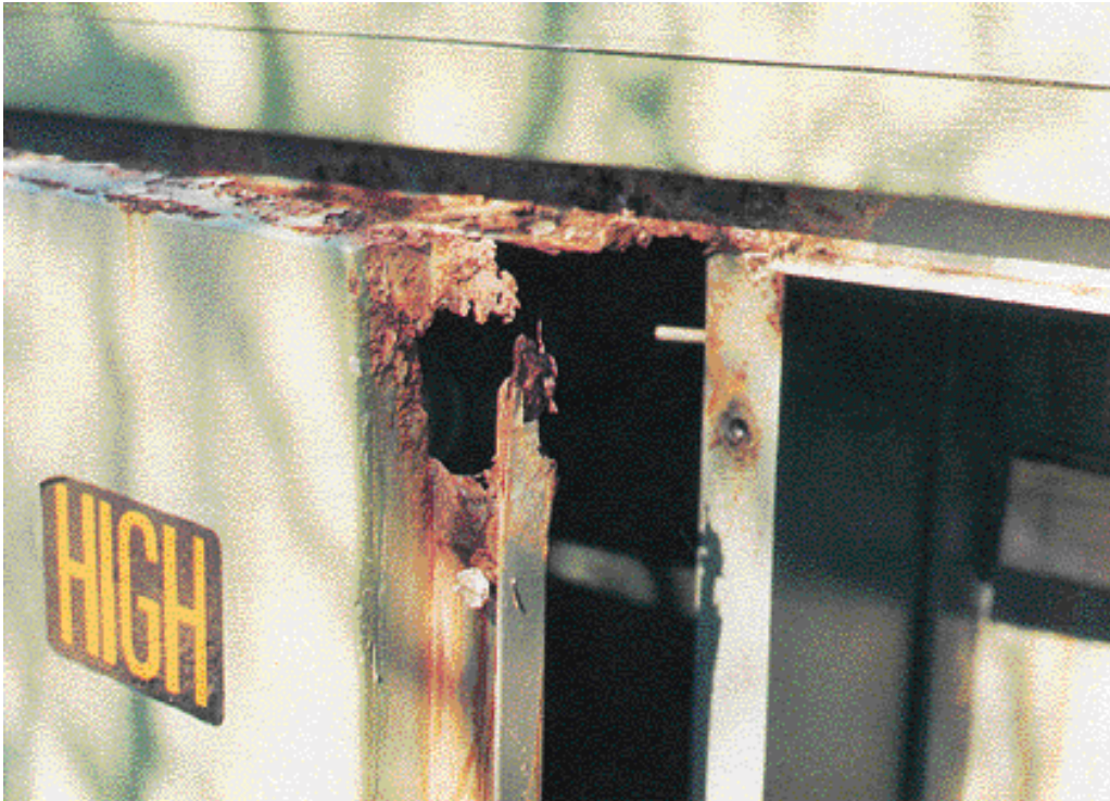
Figure 6-4: Wall Corrosion at Top of Compartment Door, Covered when Other Door Closed
