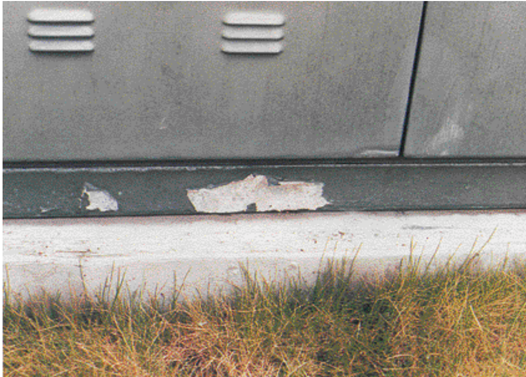
Figure 6–26: Limited Peeling of Paint
