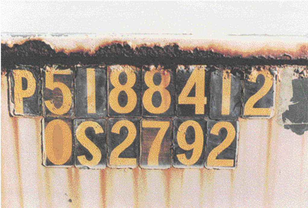
Figure 6–14: Moderate Corrosion with Pitting on Edge of Enclosure Top
