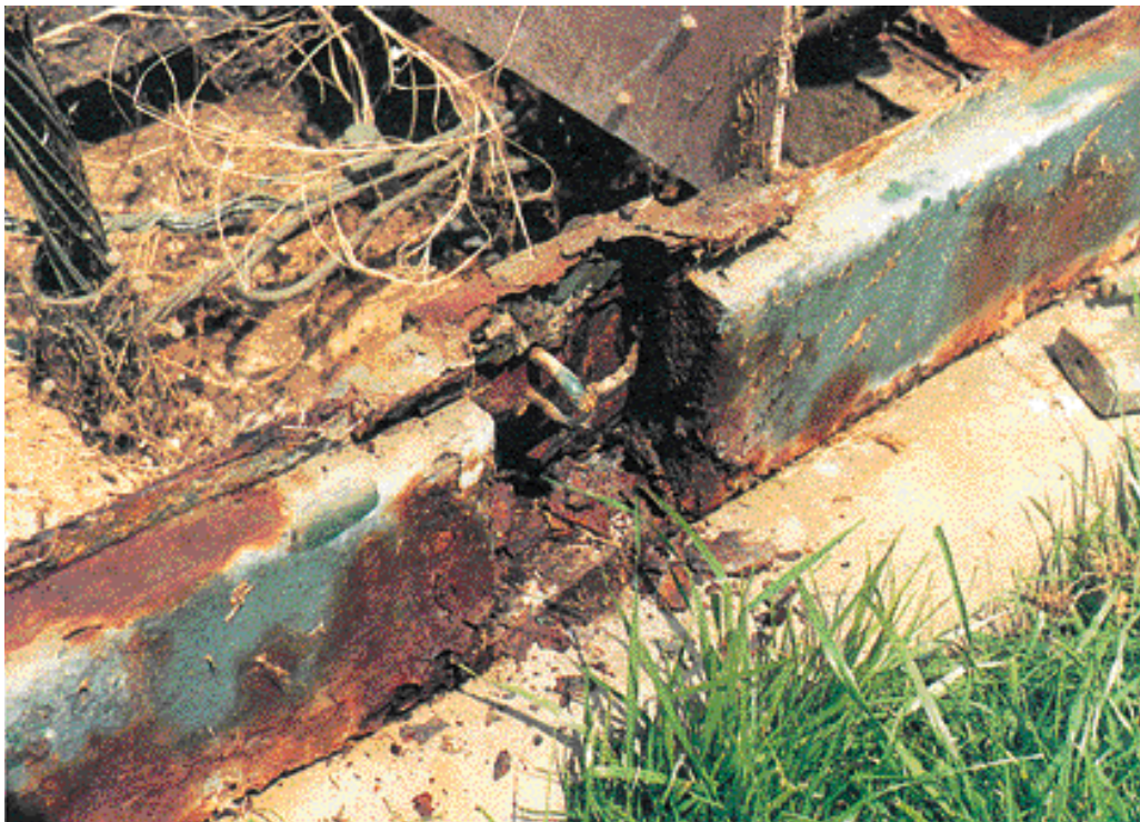
Figure 6–2: Very Heavy Corrosion of Locking Assembly
