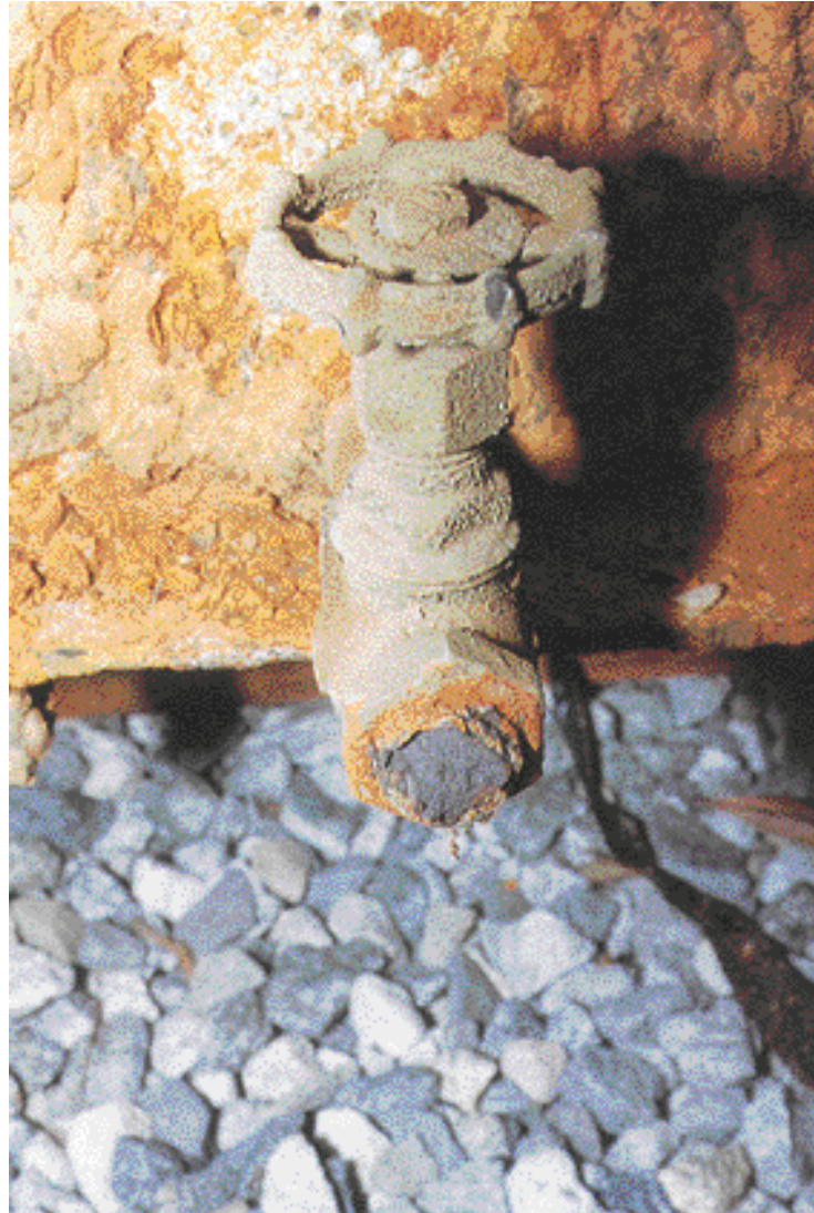
Figure 5–17: Typical Problems — Example 1 of 4
