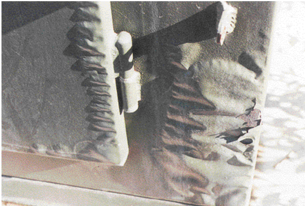
Figure 6–13: Significant Blistering of Paint
