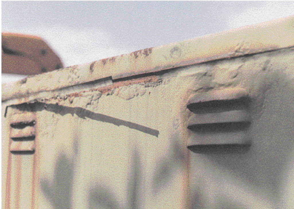
Figure 6–16: Moderate Corrosion with Blistering, Pitting, and Discoloration in and around Vents
