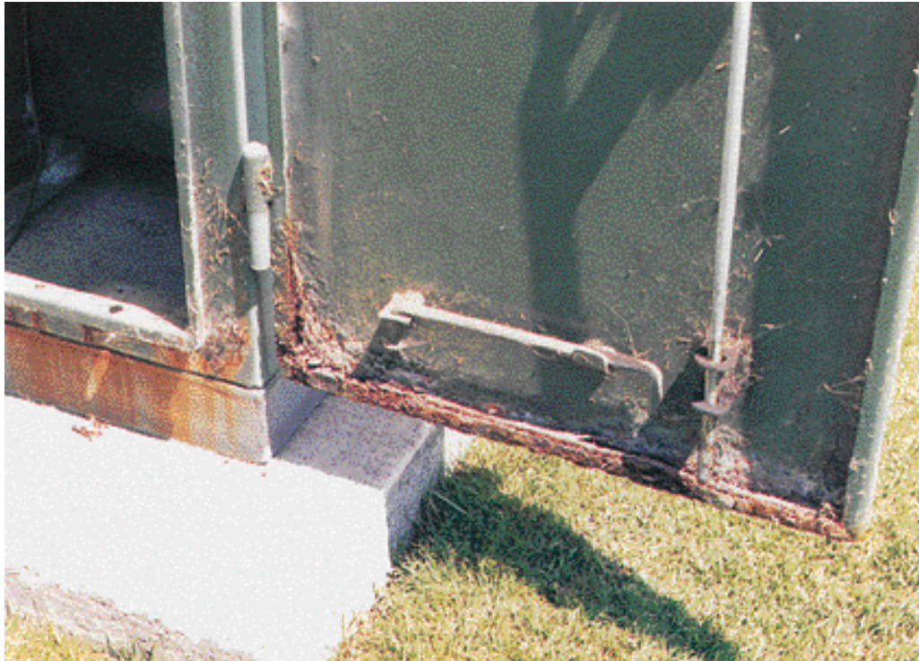
Figure 6–19: Interior Blistering, Flaking, Corrosion, and Discoloration
