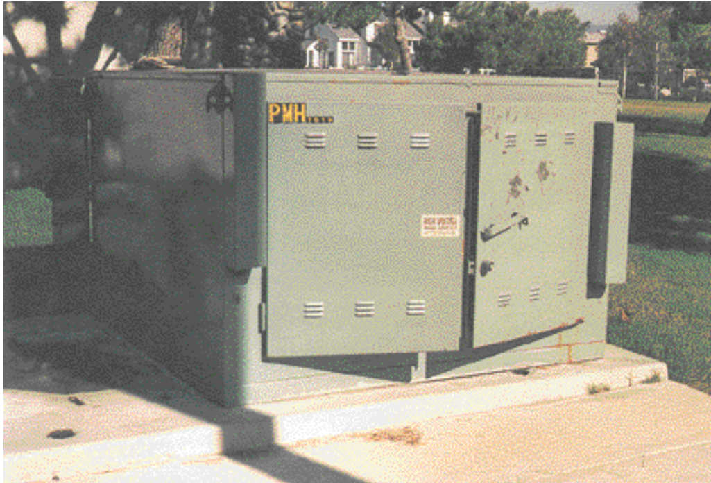
Figure 6–22: Light Corrosion on Bottom of Door (No Serious Pitting)
