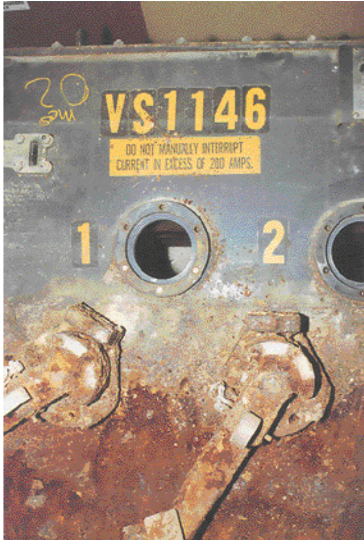
Figure 5-7: Moderate Corrosion — Example 1 of 3
