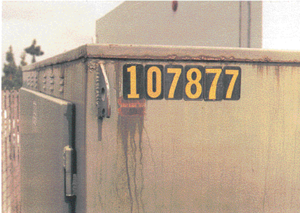
Figure 6–28: Light Corrosion at Lower Edge of Top Cover and Brackets (No Serious Pitting)
