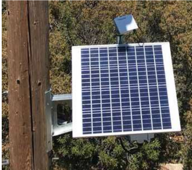
Figure 1125–3: Typical Installation of Weather Monitoring System (NEMA Enclosure and 60-Watt Solar Panel)
