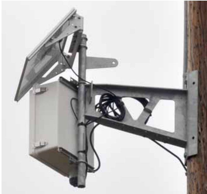
Figure AP 810–5: Typical Installation of Weather Monitoring System (NEMA Enclosure and Solar Panel) — FRO
