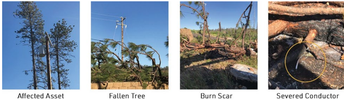
Figure F-2 PG&E Covered Conductor Effectiveness – Example 1
