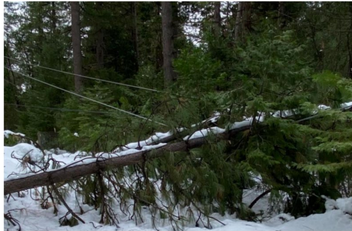
Figure F-4 PG&E Covered Conductor Effectiveness – Example 3
