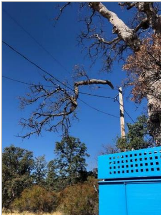
Fig. 67. Example of branch blown into electric line
