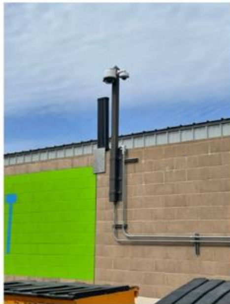
Figure TBC 8.1.2- 1. Perimeter Wall and Cameras
