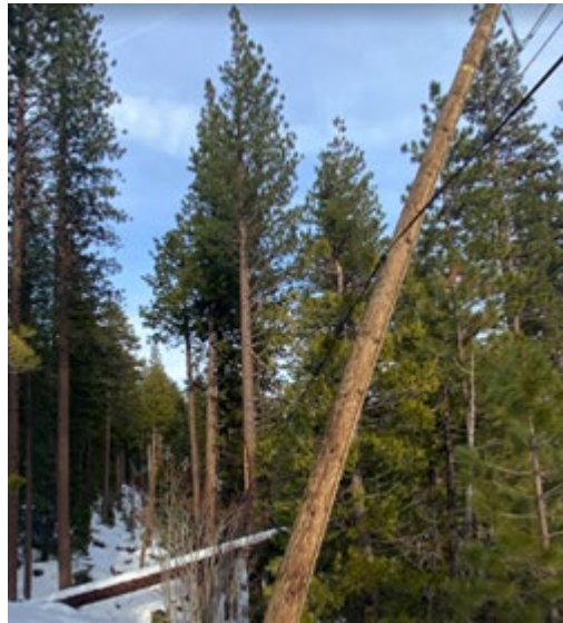
Figure F-7 Liberty Spacer Cable System Preventing a Fault – Viewpoint 2
