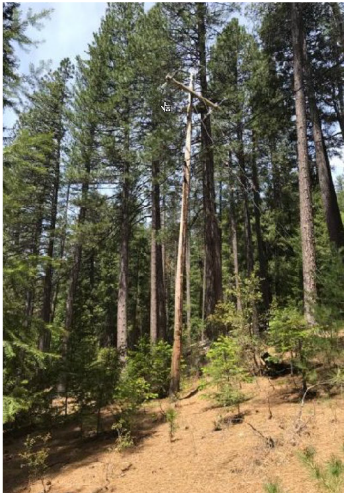
Figure 7 SAP Pole ID 100111818 taken on May 14, 2019, by WSIP inspector.
