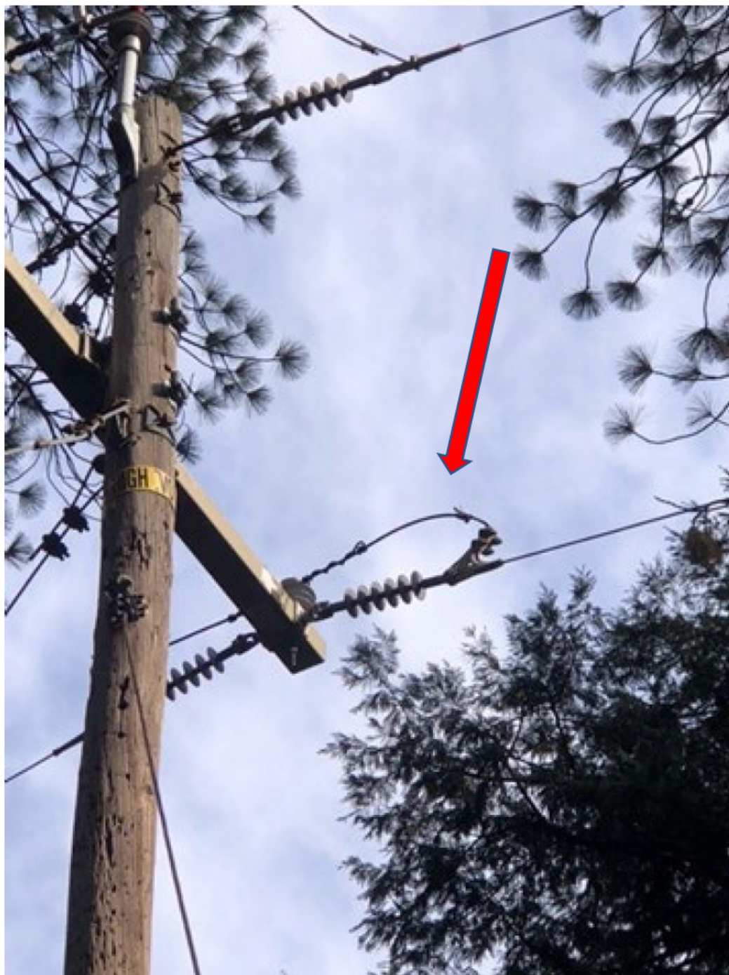
Figure 5 SAP Pole # 100111818, photo taken by troubleman on April 18, 2022, the arrow pointing at the location where the bad connector was located before failing.
