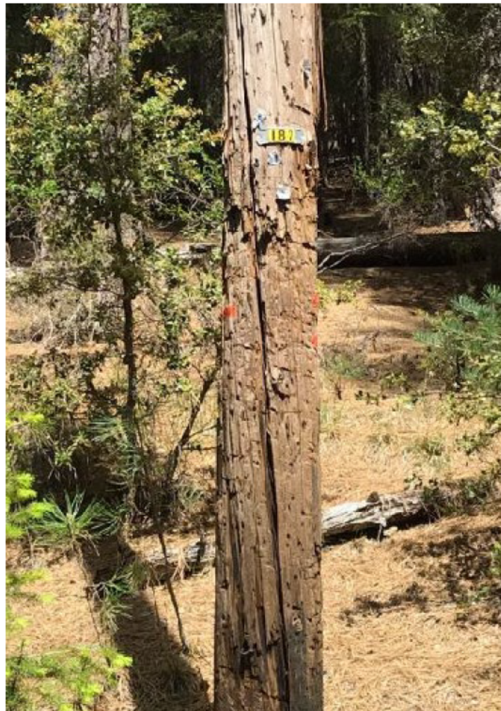
Figure 8 SAP Pole ID 100111818 (showing animal damage) taken on May 14, 2019, by WSIP inspector.
