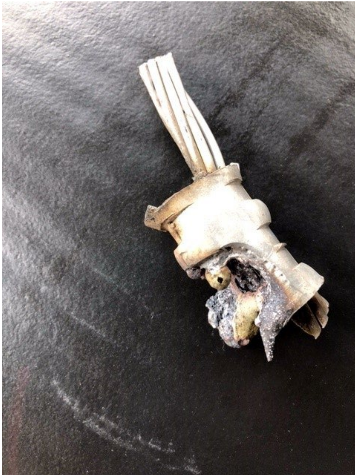
Figure 6 Photo of faulty/bad connector taken on April 18, 2022, by the responding troubleman.
