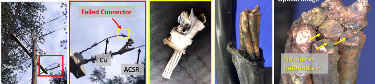
Figure 11 Visuals from analysis performed by ATS on the failed compression connector.
