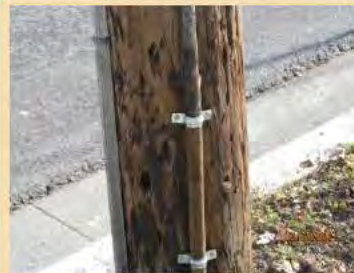
At this Location: Condition acceptable after repair with wood molding
