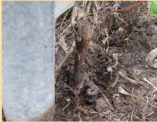
Anchor above ground
