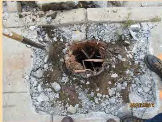
After extraction showing below ground deterioration
