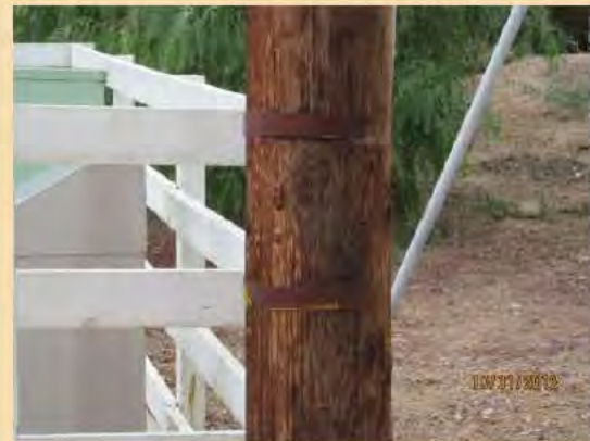
At this Location: Visibility strips painted brown (3 rd visibility strip located above not shown in picture)
