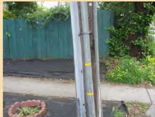
At this Location: Pole with vehicular exposure. Two small sections of yellow adhesive visibility strips.
