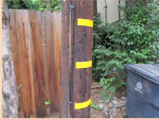
At this Location: Acceptable metal visibility strips attached 1 ½" from ground.
