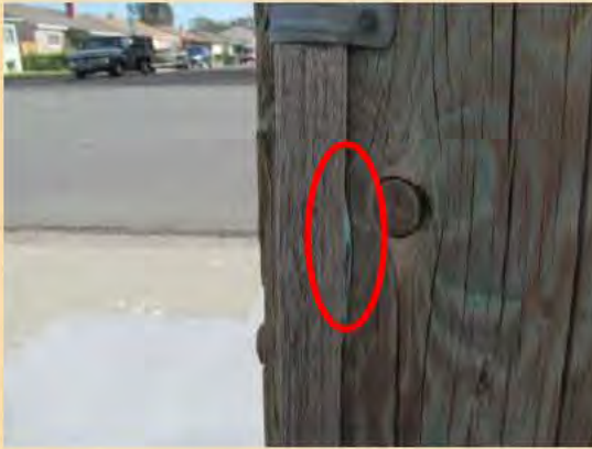
Before: Copper Wire sticking out from under the wood molding
